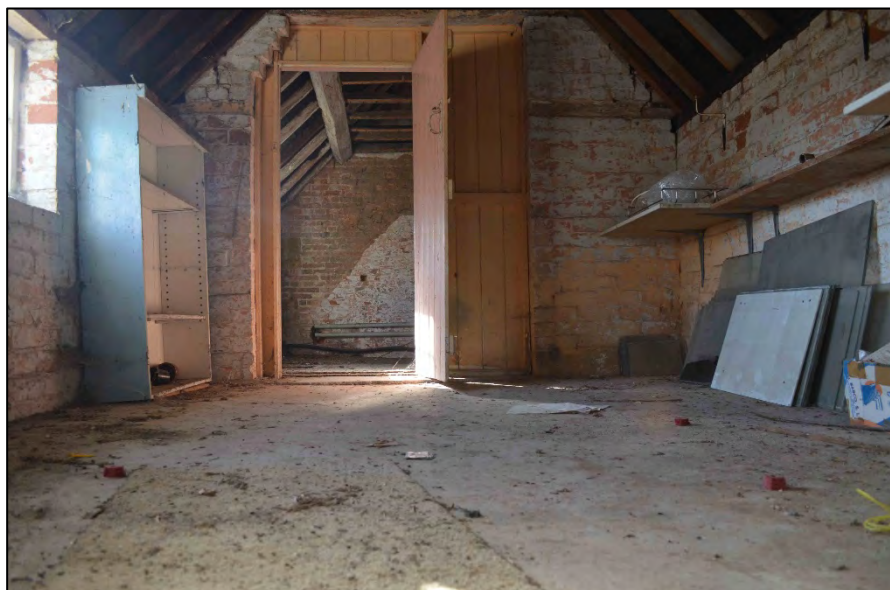
Appendix 2.31: View looking through F11 to F10, noting gable scar on far wall of the Hall
