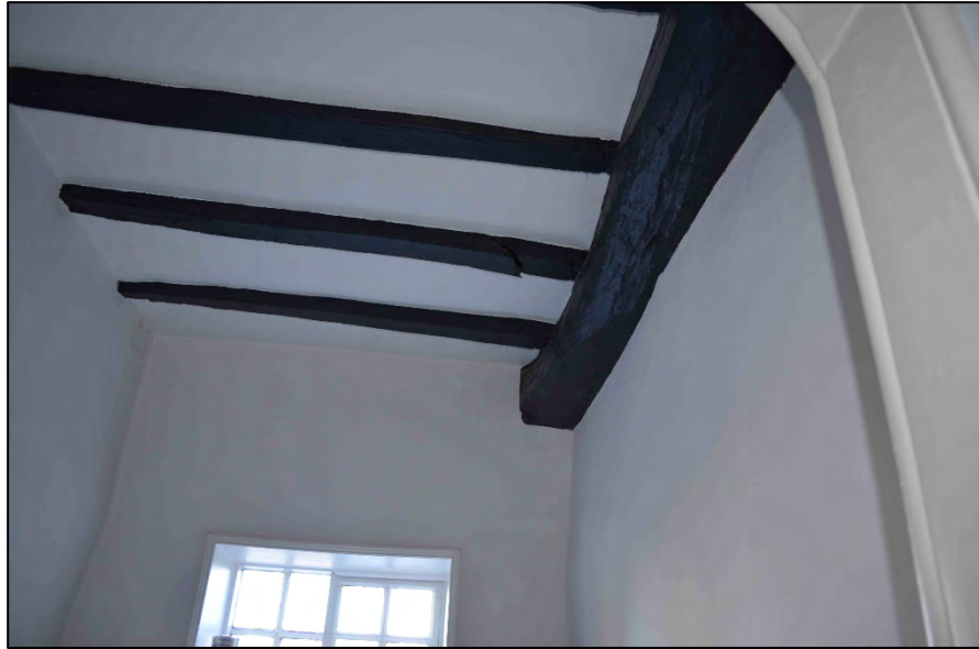
Appendix 2.23: View of beam above wall between F7 and F8, looking north
