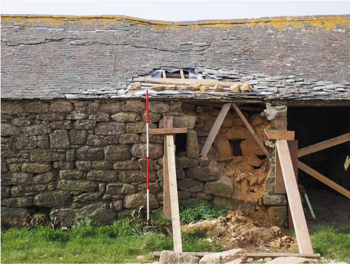
Figure 58: Cartshed NE wall showing collapsed section
