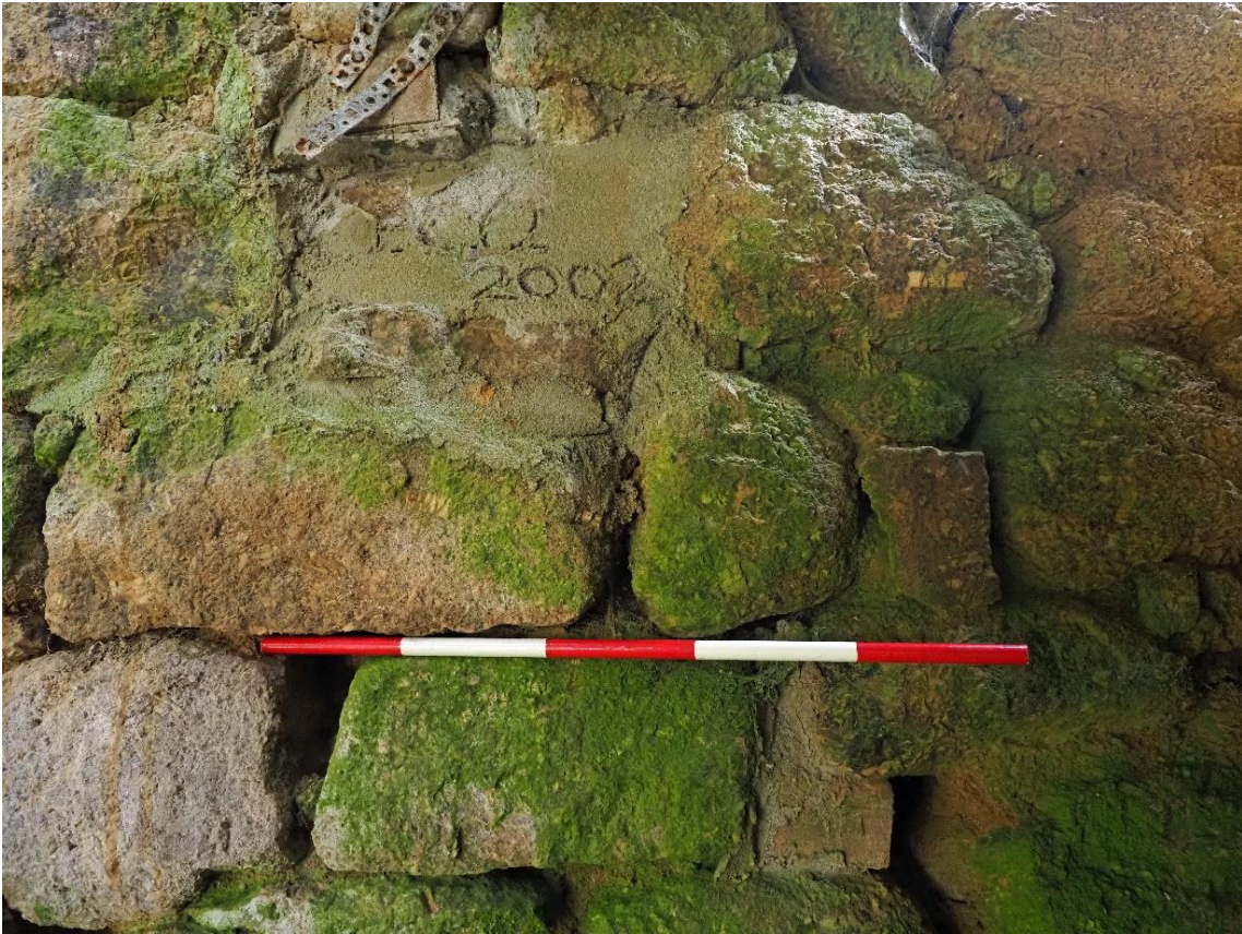
Figure 52: Cartshed SE wall: inscription in mortar repair: EOO 2002
