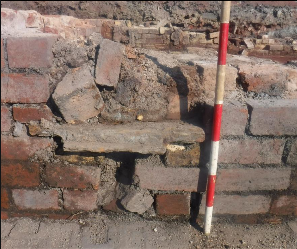
Plate 11. Flue vent in western wall of Kiln B showing iron base plate, looking east.
