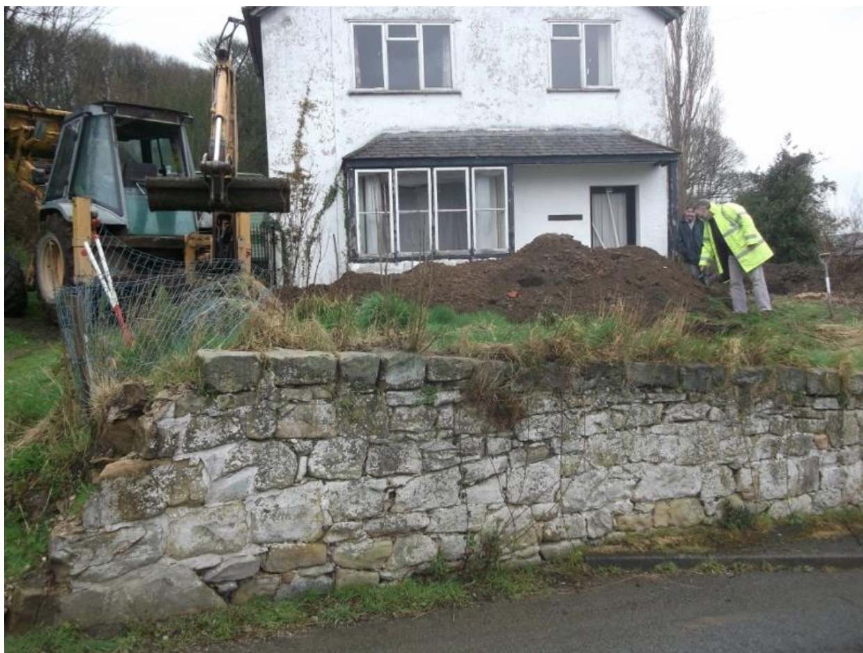
Figure 11 East facing shot, showing location of trench 1, and relative height of retaining wall facing Llwyn Road
