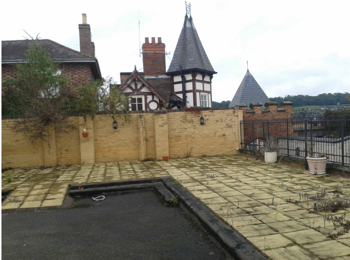
Figure 11 interior view of Castle Terrace wall showing cracking and buttresses to wall
