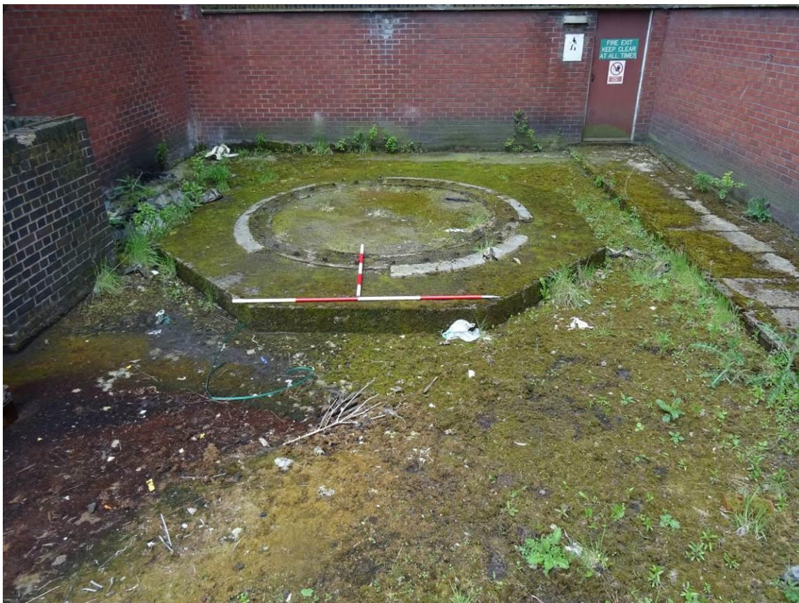
Plate 62. Chimney base located within the western recess within the rear section of the building
