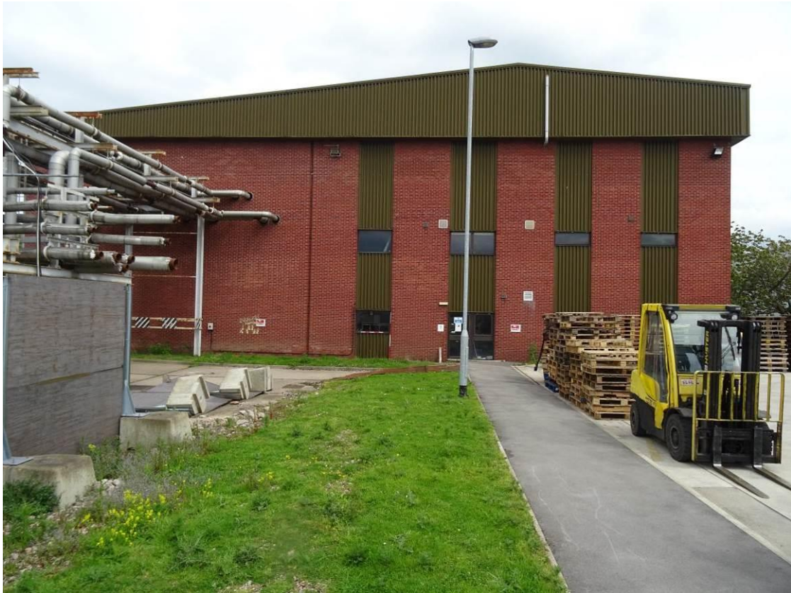
Plate 53. SW view of the Boiler House showing an array of pipework extending from the rear section of the building, initially providing heat for the site
