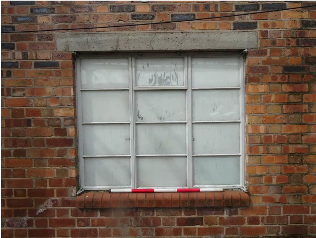
Plate 32. Detail showing a window casement incorporated into the NE elevation – see Plate 30
