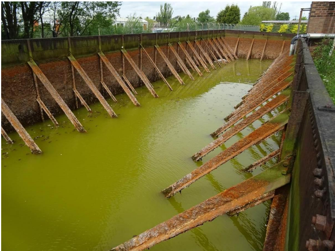
Plate 29. Stagnant water within the earlier filtration tank, looking NW
