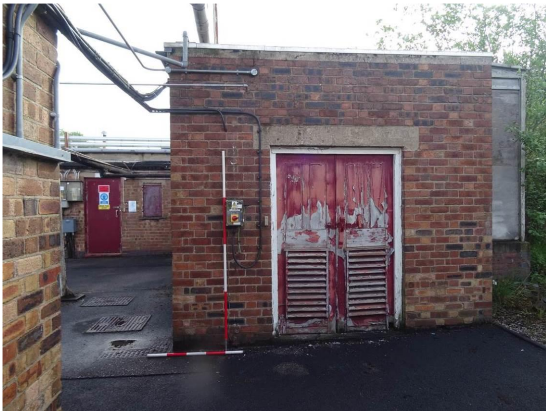
Plate 6. Electrical transformer building (C), located outside the main Firing Range Complex, looking west
