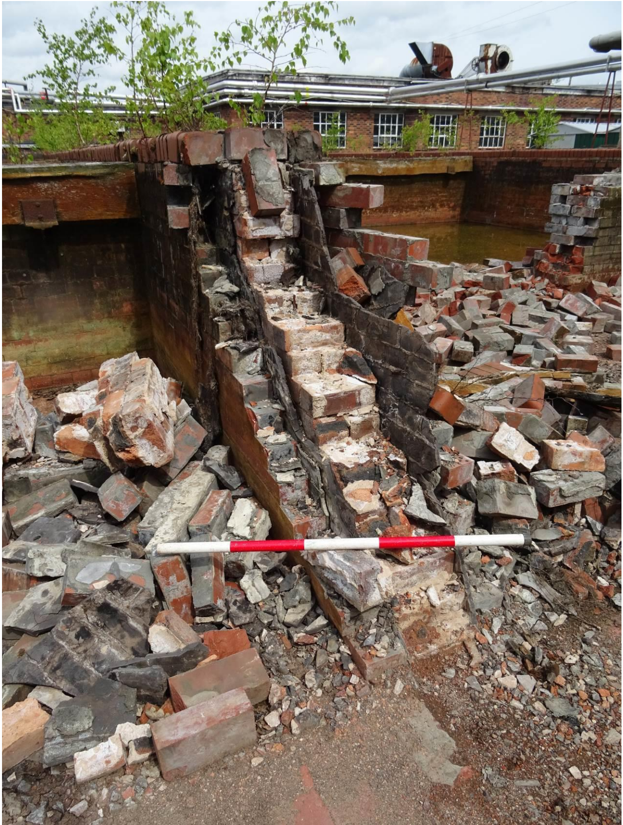
Plate 27. Destroyed internal brick wall revealing the brick and slate construction, looking north
