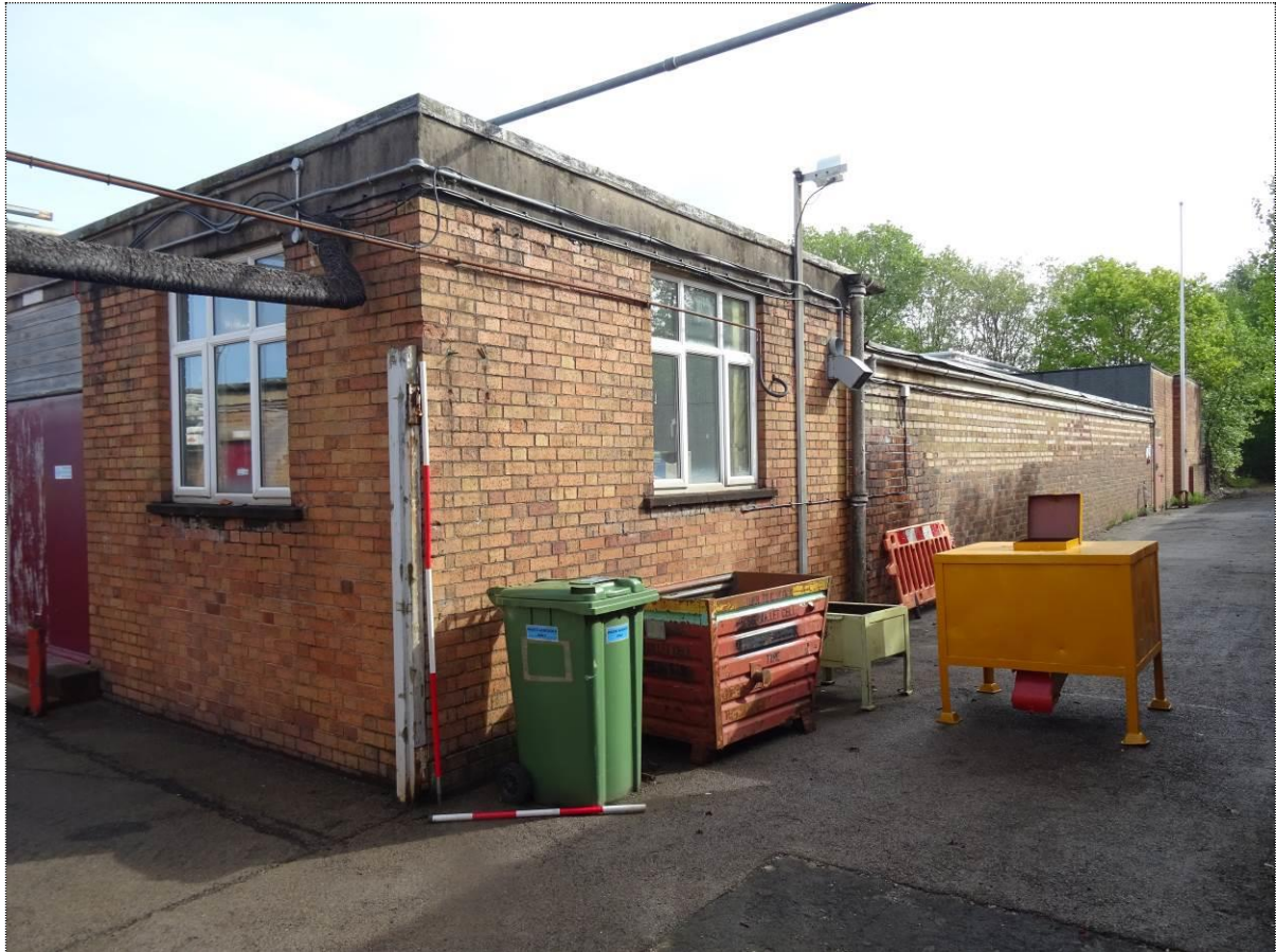
Plate 9. NE view of the southern section of Building E, showing the southern elevation (see Plate 10)
