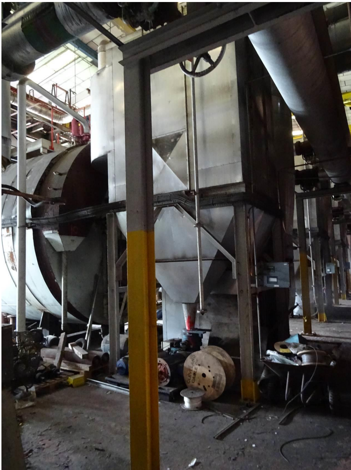
Plate 65. Steel hoppers located to the rear of the boiler unit
