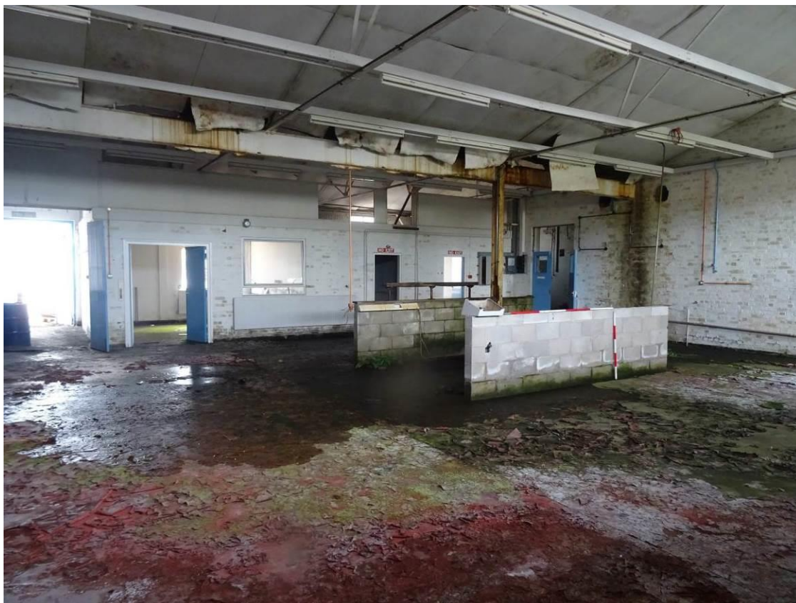
Plate 40. Internal view of one of two principal rooms – southern room, looking NE
