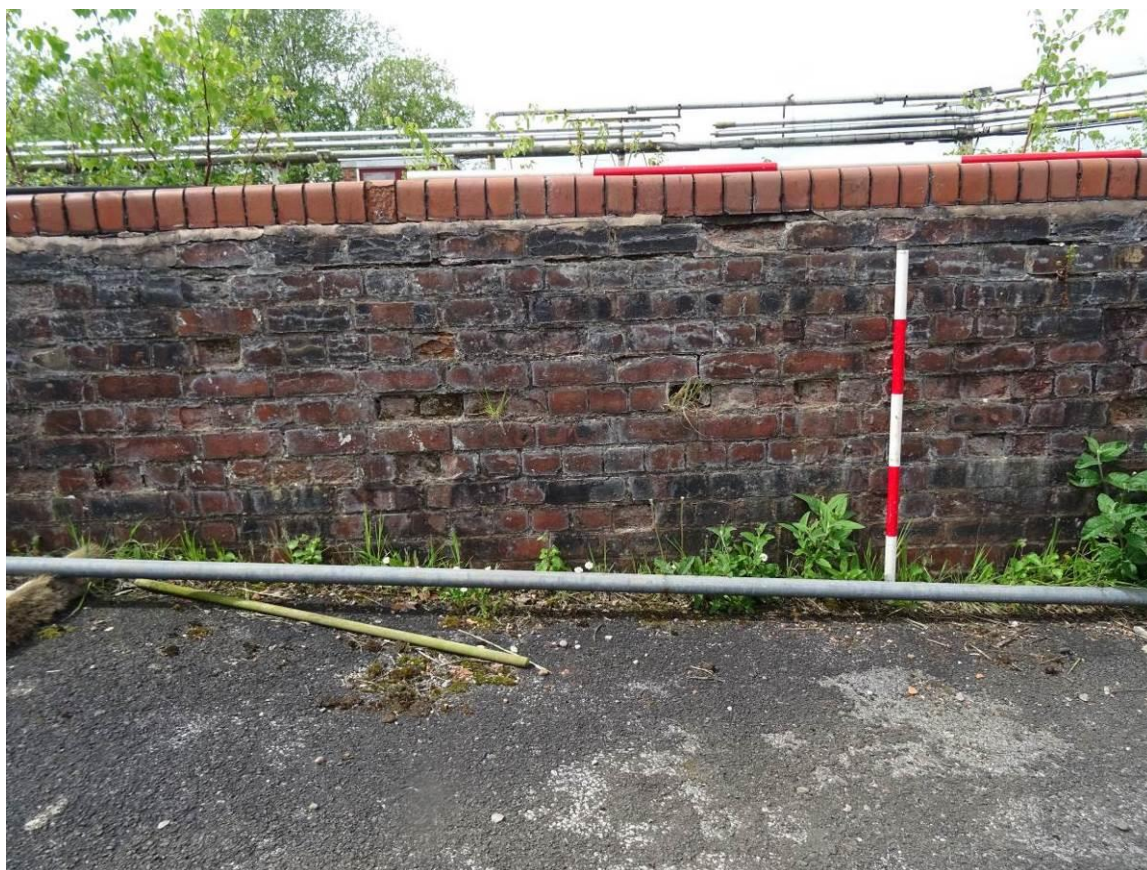
Plate 24. NE wall section of the second set of filtration tanks, looking SW
