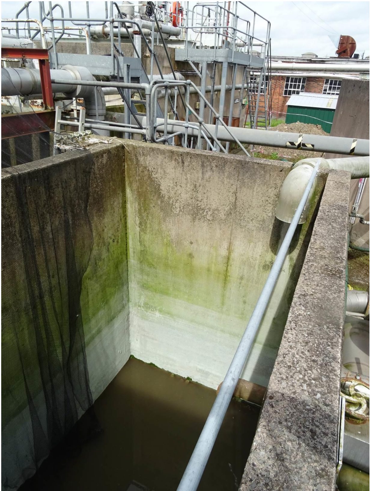
Plate 22. An above view of the sludge tank (4), looking north
