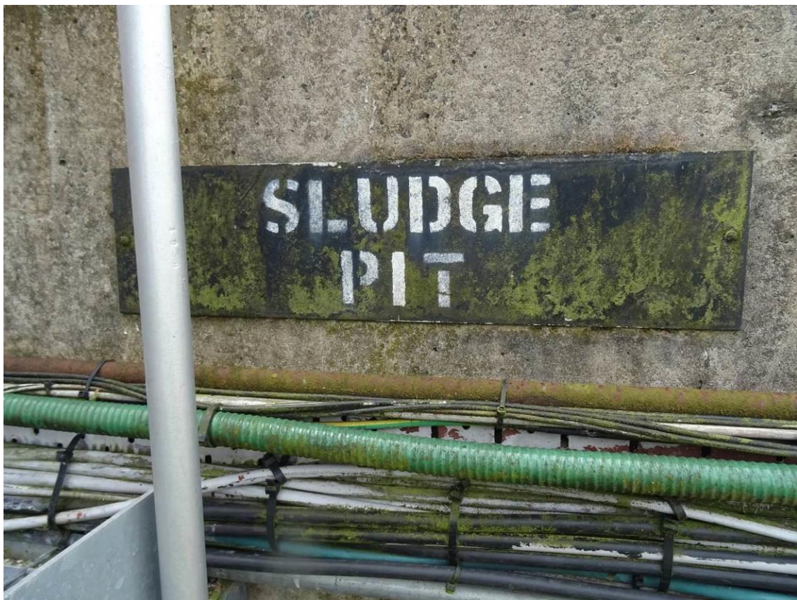
Plate 21. Make-shift signage located on the 'Sludge Tank (Building 4)' (see Plate 20)
