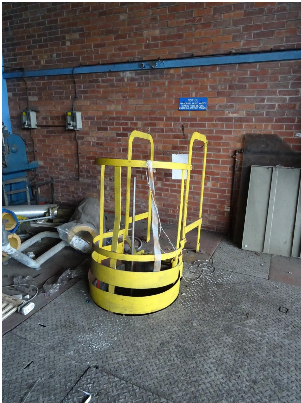
Plate 68. One of two subterranean access stairwells leading to maintenance areas beneath the boiler units
