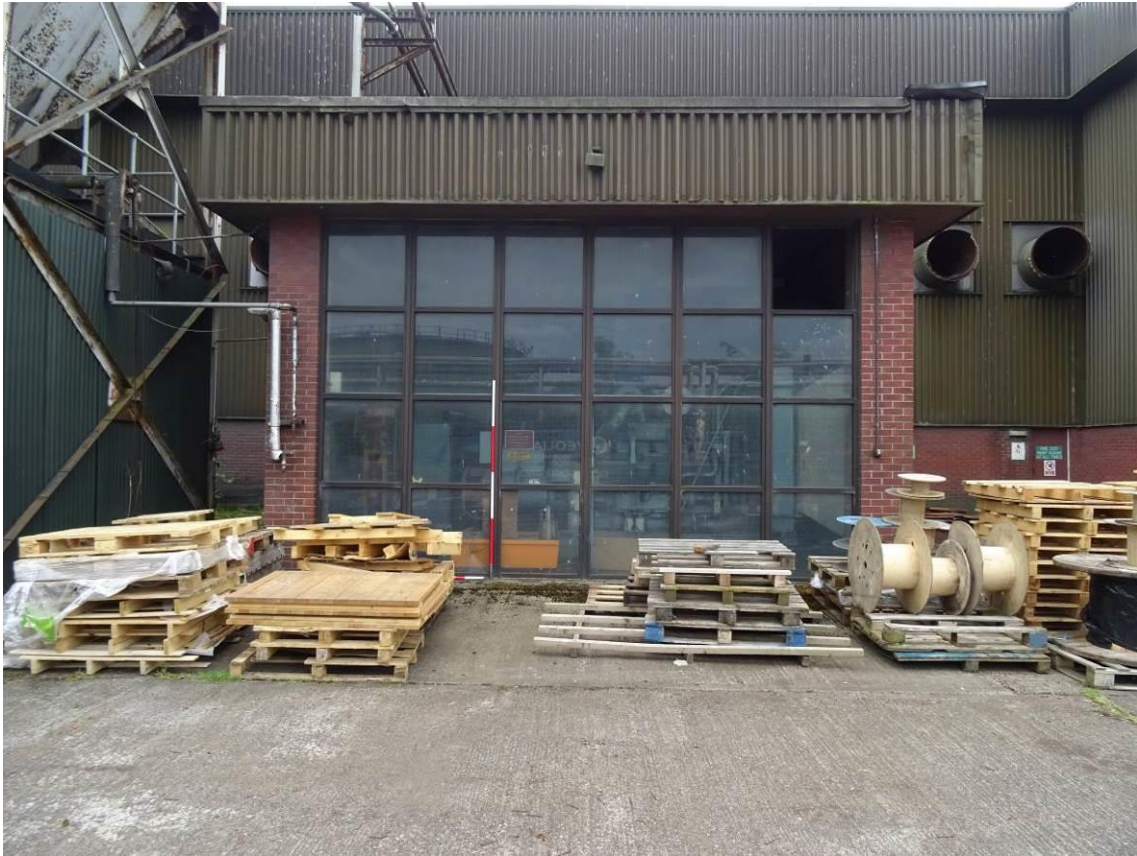
Plate 61. One of the recessed rear sections of the diesel generating and compressor facility building, looking SE
