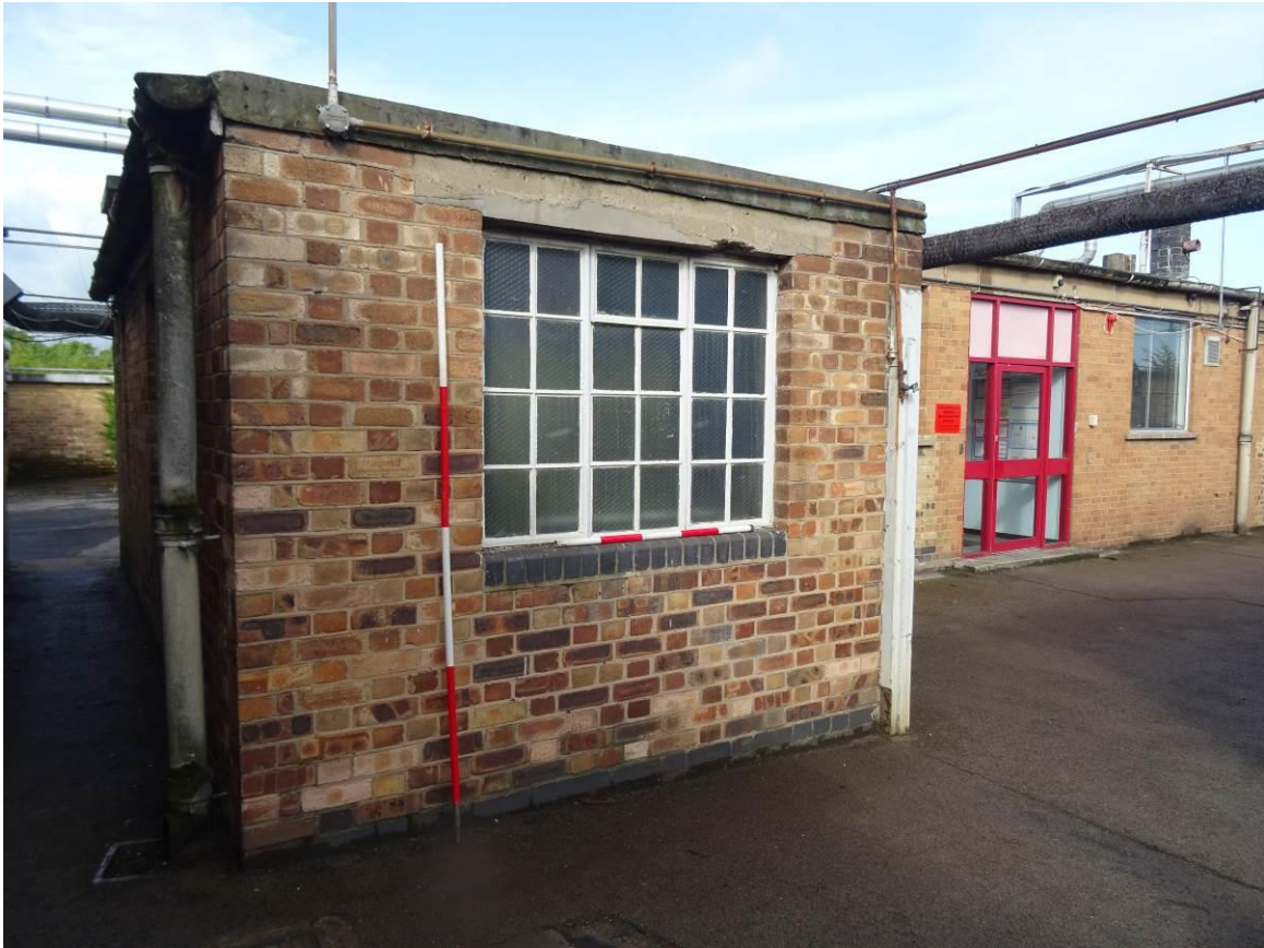
Plate 7. Rear western section of the reception building (image taken within the enclosed courtyard of the main Firing Range Complex), looking west
