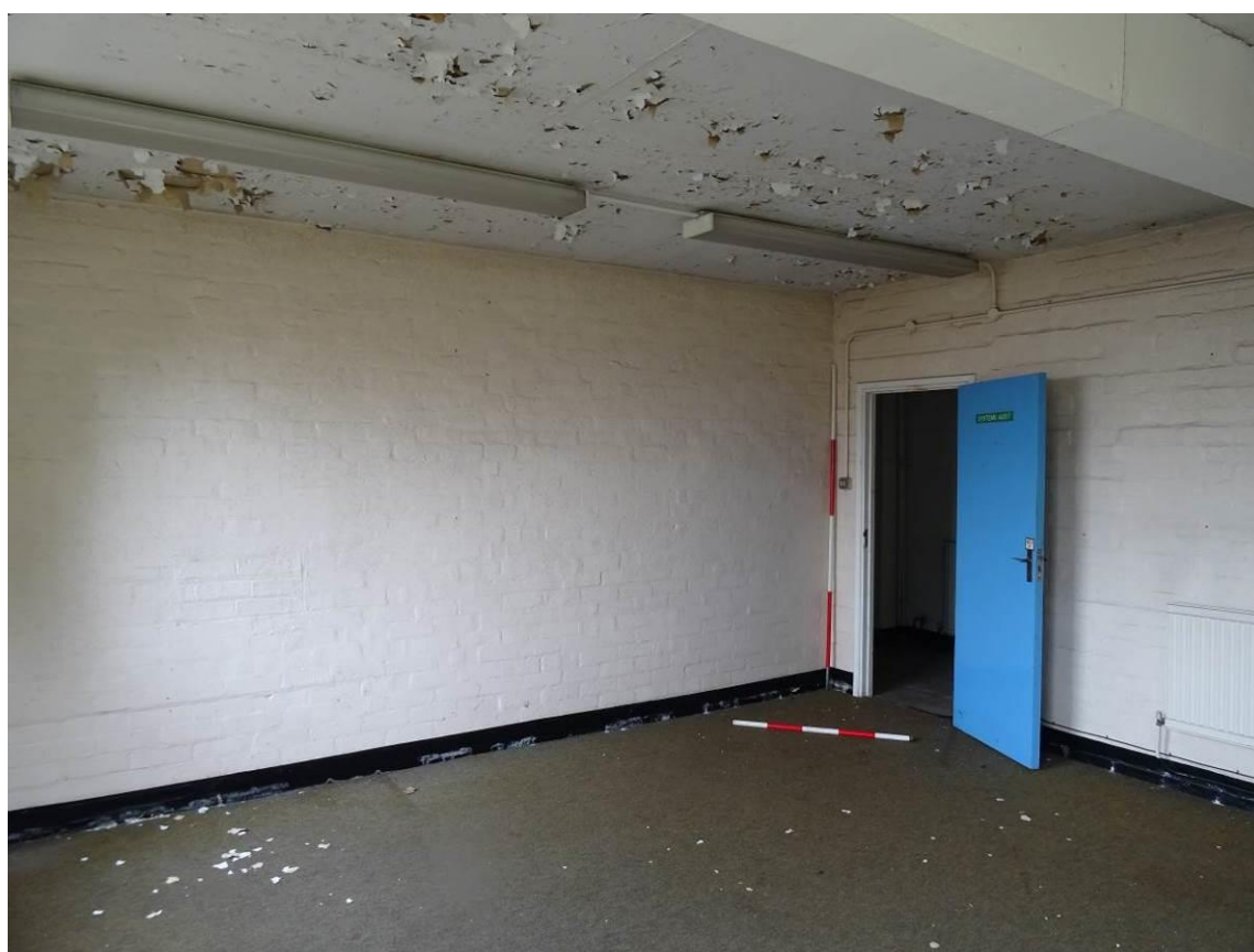
Plate 50. Systems Audit Room, located within the western [office] section of the building
