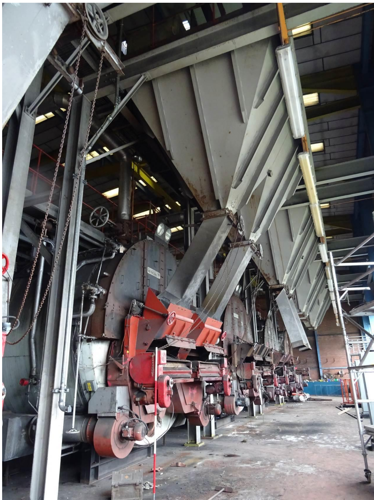
Plate 64. The row of Danks of Netherton coal-fired boilers located within the principle room of the boiler house
