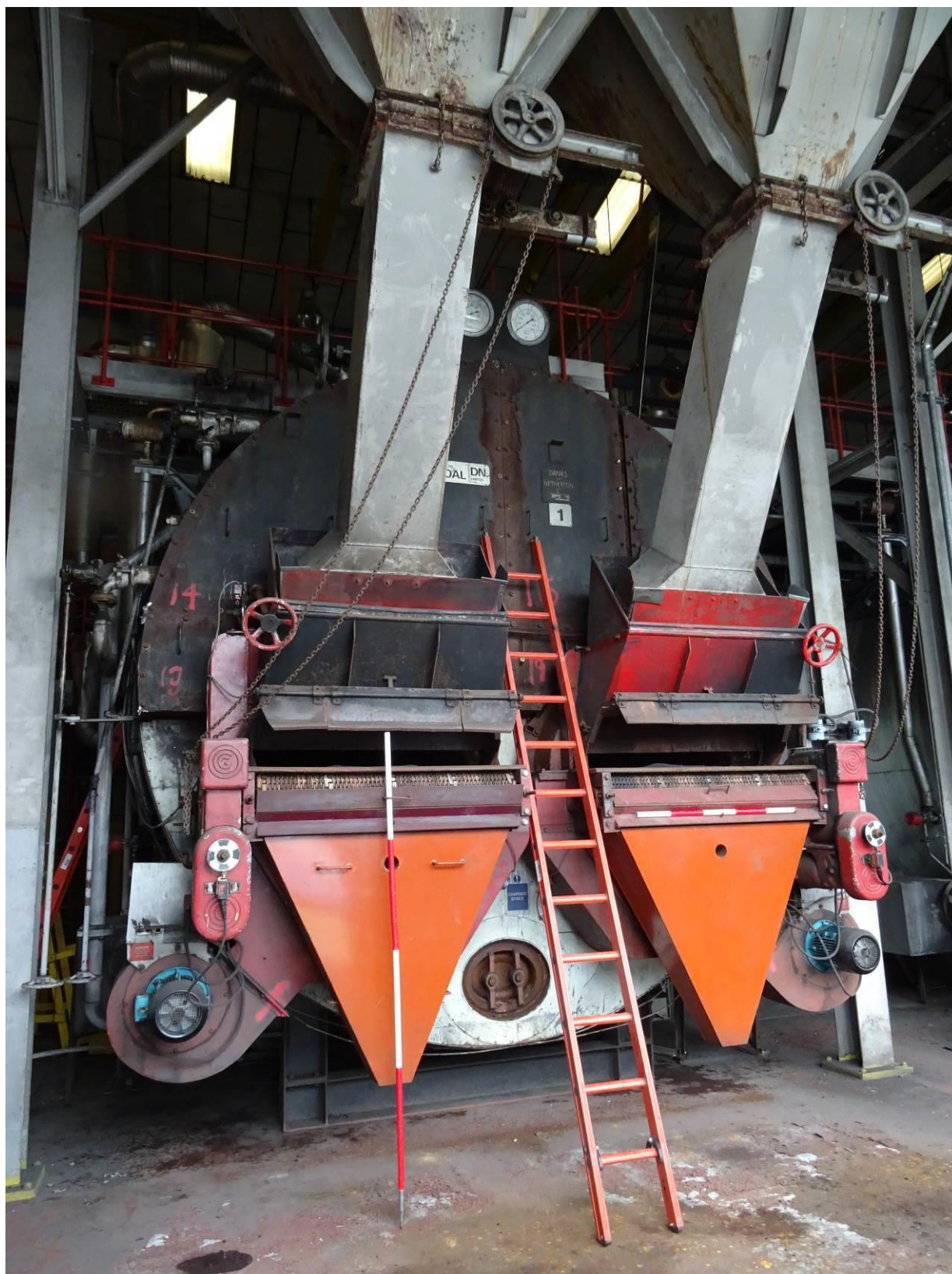
Plate 63. One of five cylindrical boilers located within the principle room of the boiler house
