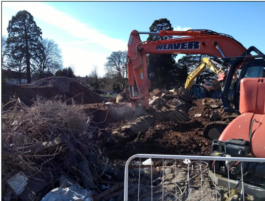
Figure 16 Removal of footings at south of former police station looking south west
