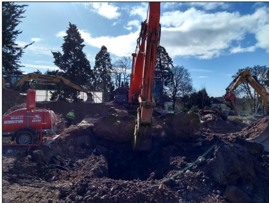
Figure 17 Removal of footings towards eastern end of former police station site looking south
