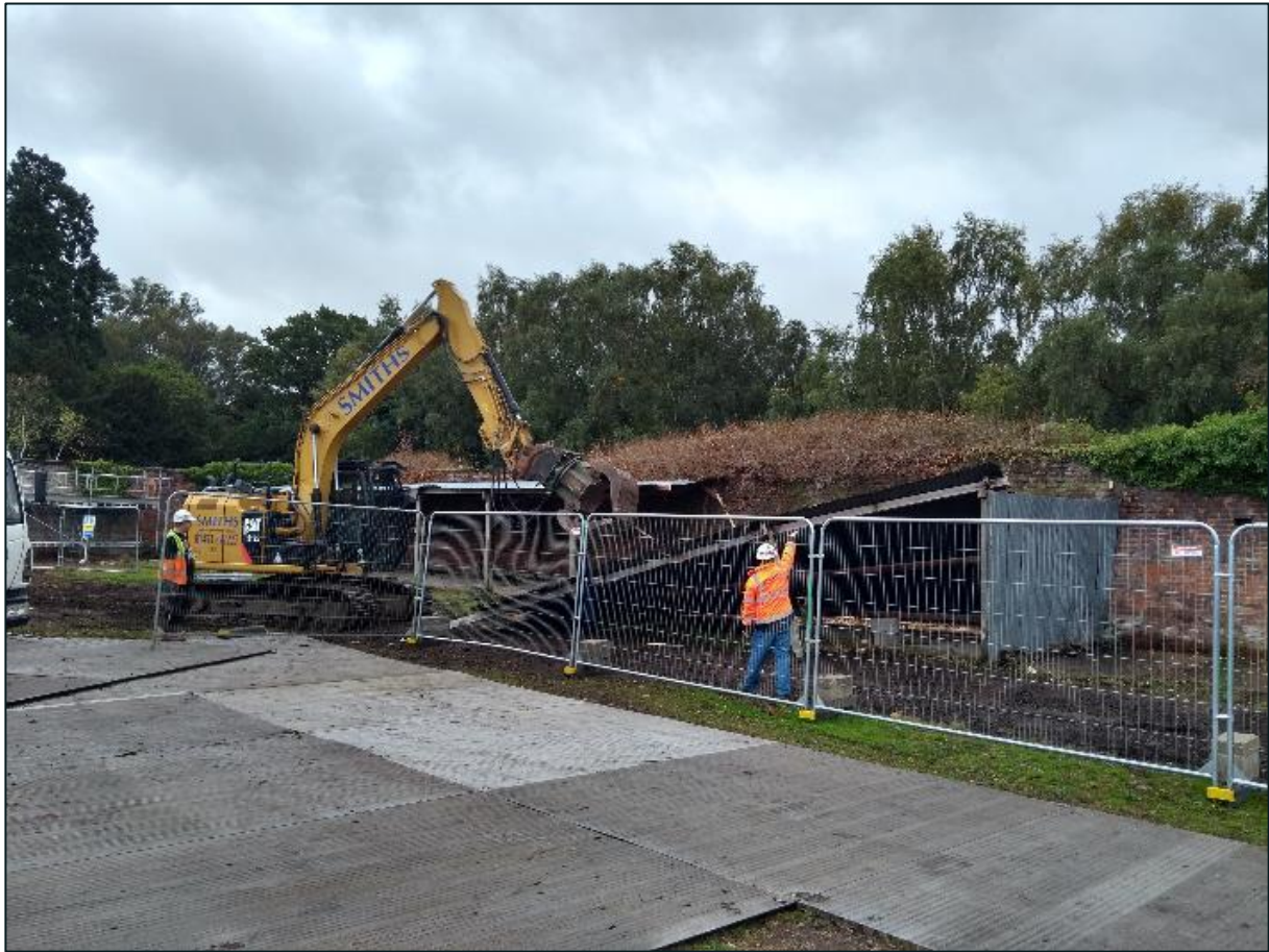
Figure 3-2 Removal of lean to structures at south east of site looking south east
