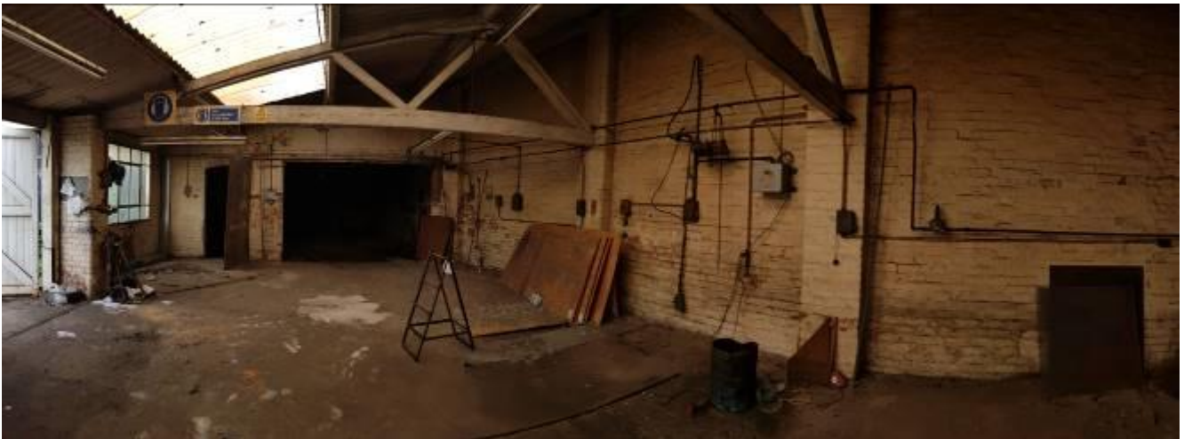
Plate 47: Section D view south. Section B is located at the far room. Panorama, no scale.
