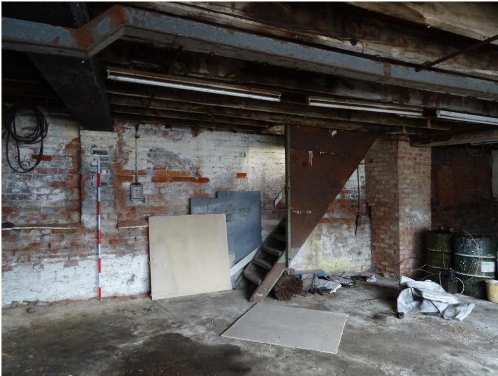
Plate 36. Southern elevation of section B with staircase to upper floor C. 2m scale.
