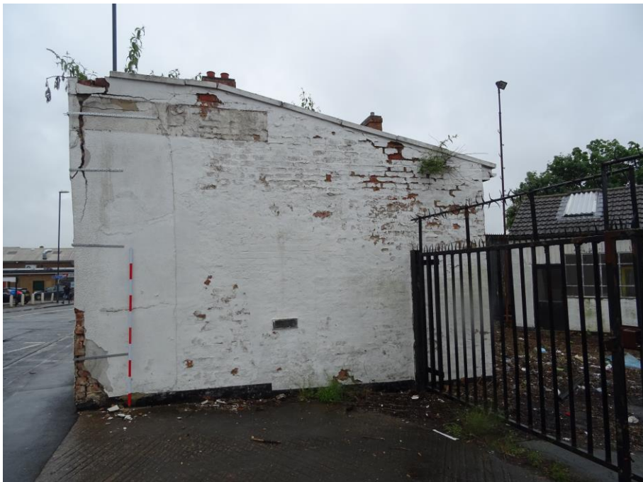
Plate 7: front entrance off Mansfield Road. Iron railings of site compound to right of the image. 2m scale.
