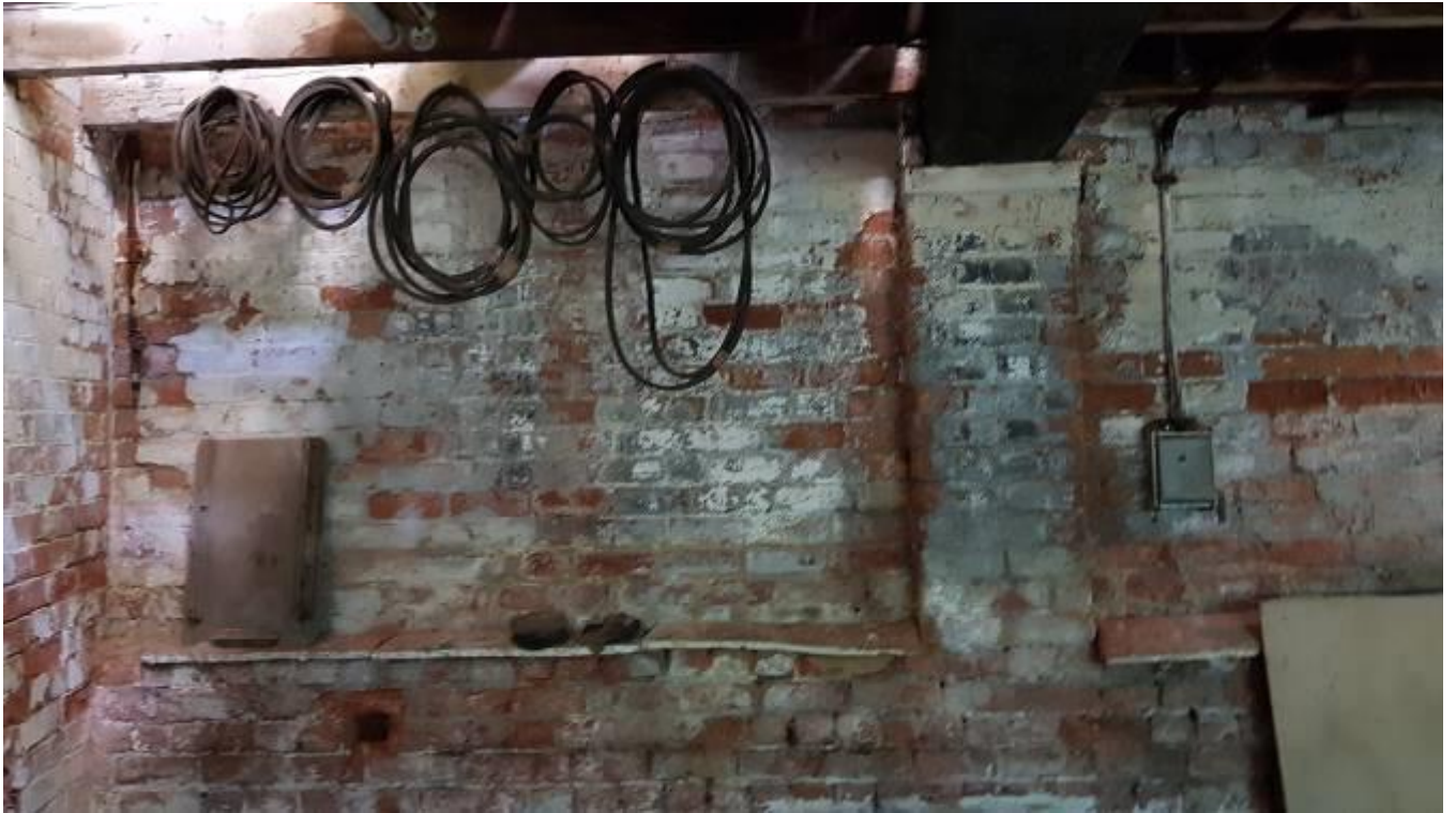
Plate 38: internal of southern exterior wall section B. No scale.
