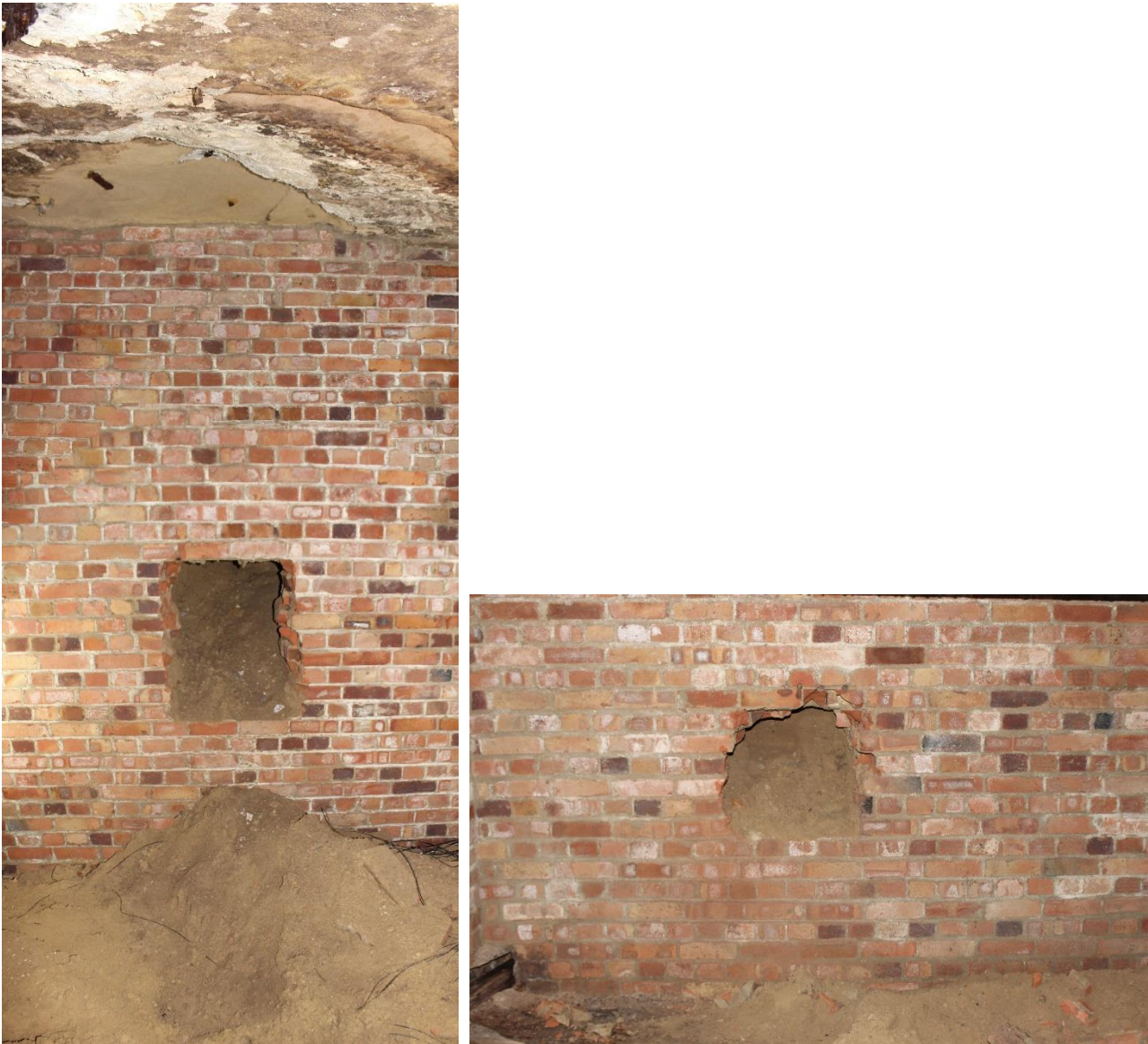
Figure 4-20 Openings at the Northern (left) and Southern Ends of the 'Destroyed Caves'
