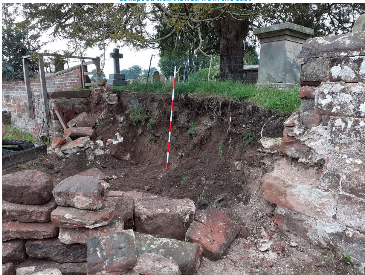
Figure 7 Collapsed wall viewed from the east
