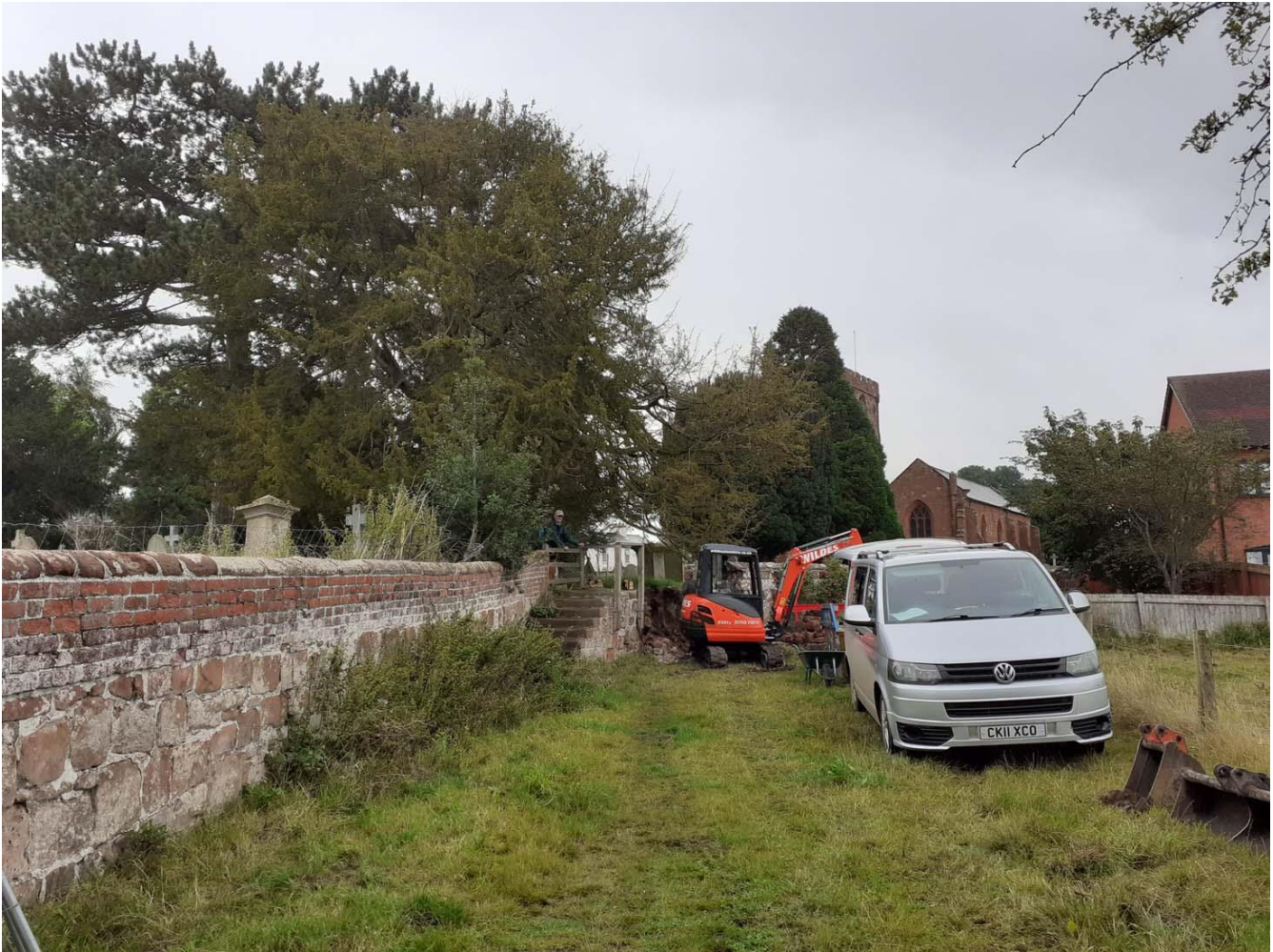
Figure 4 View towards collapsed wall from south-west with church in background
