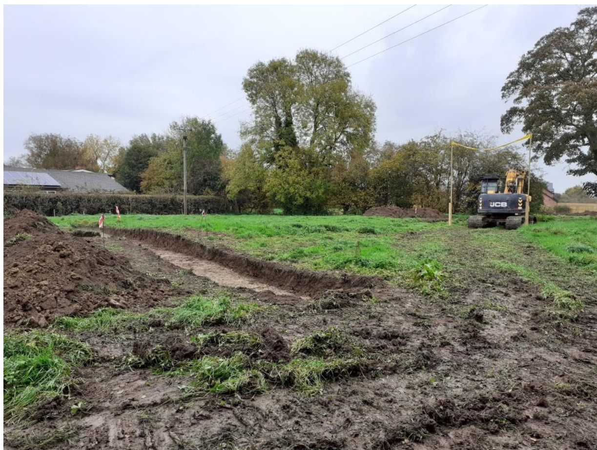
Figure 2-4 View of middle field with Trench 4, beneath ridge or relict headland, looking north
