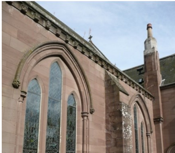
Illus. 64: South elevation of the nave of Brechin cathedral (© Copyright 2013, SCHR Ltd. All rights reserved).
