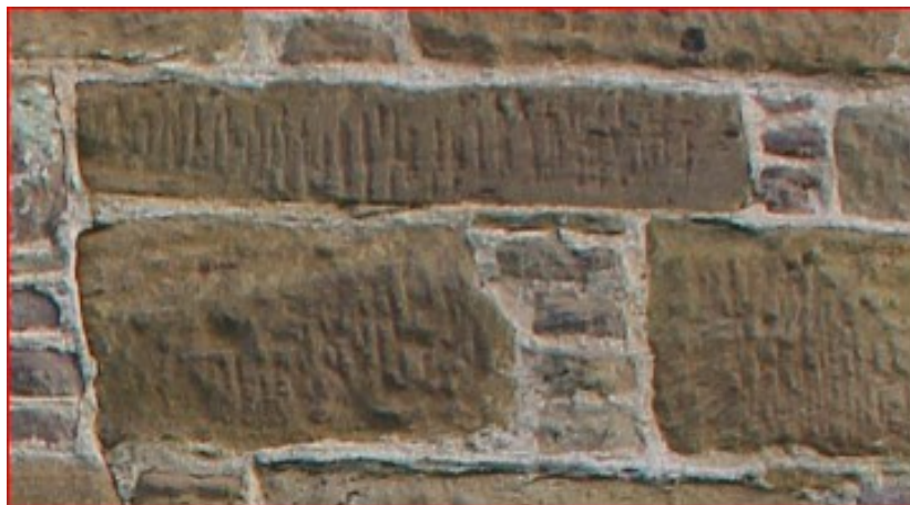
Illus. 12: Stonework detail on part of the west gable, with evidence of possible harling.
