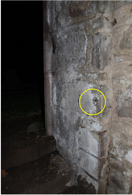
Illus. 54: Hole in doorway 006 (north wall).
