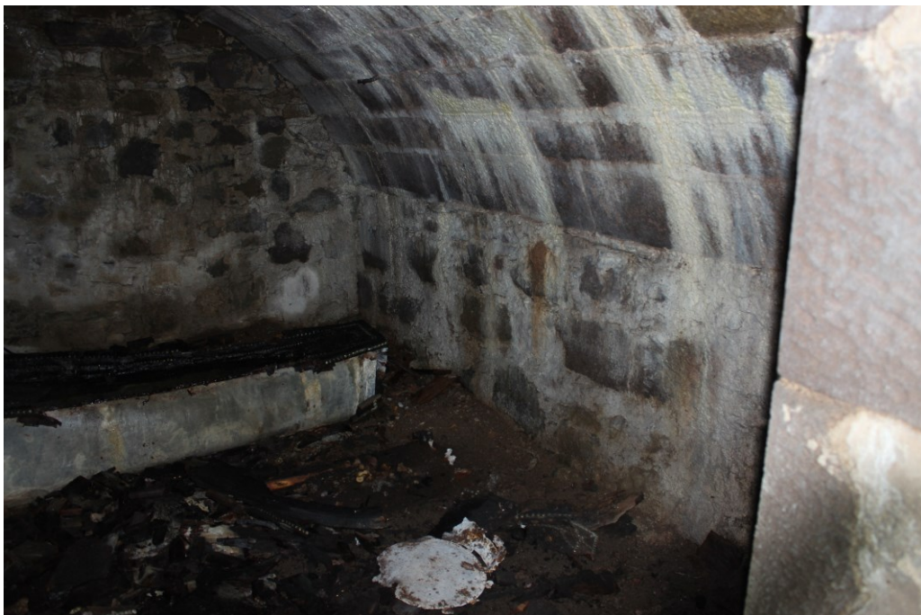
Illus. 60: View of barrel vault 060 , showing clearly that it is an inserted feature.
