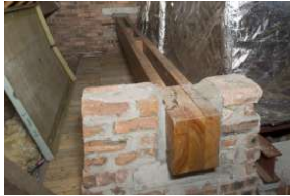
Figure 48: The 'hanging beam' located in the attic of the execution chamber (Fig.11, location 22) (dp_172954 - RCAHMS)
