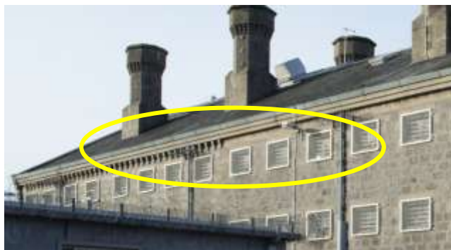
Figure 12: A change in building construction seen on the eastern elevation of 'A' Hall (DP_172931 - RCAHMS)
