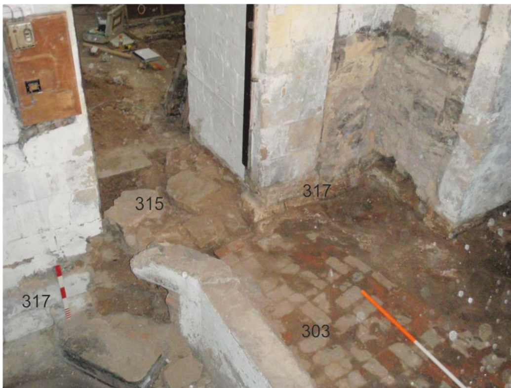
Pl. 64 Tower door threshold after removal of concrete steps, looking south-east. Scales 1 and 0.50m
