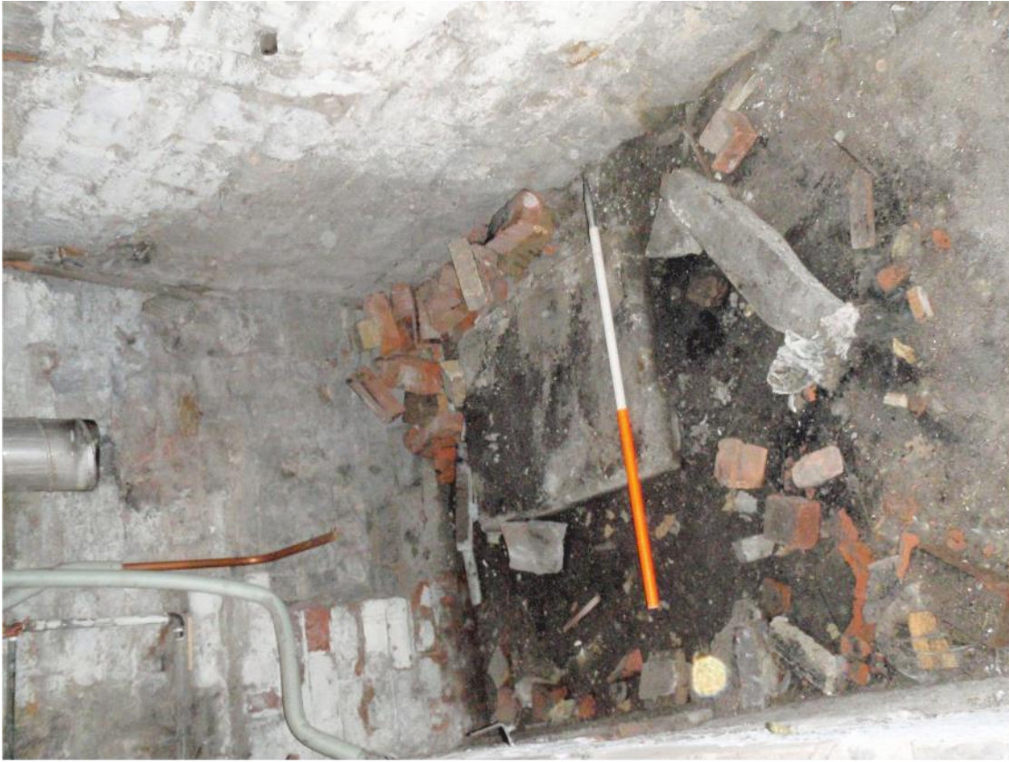
Pl. 54 Tower boiler cavity after removal of the boiler, looking north-west. Scale 1m.
