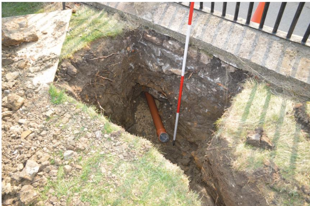
Pl. 30 Connection of pipe through the churchyard wall along Bolton Lane. Scale 2m
