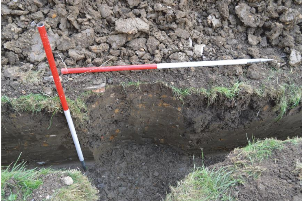
Pl. 27 Location of inspection chamber at junction of the two pipe trenches showing undifferentiated clayey soil below the turf
