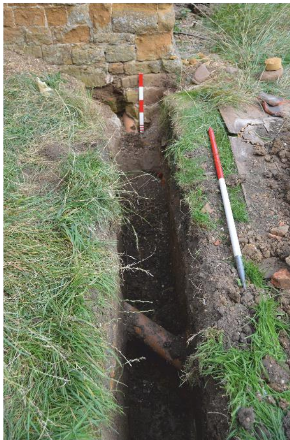
Pl. 24 Pipe trench extending west from the west wall of the south porch, looking east. Note the drainage pipe crossing the trench. Scales 1m and 0.50m
