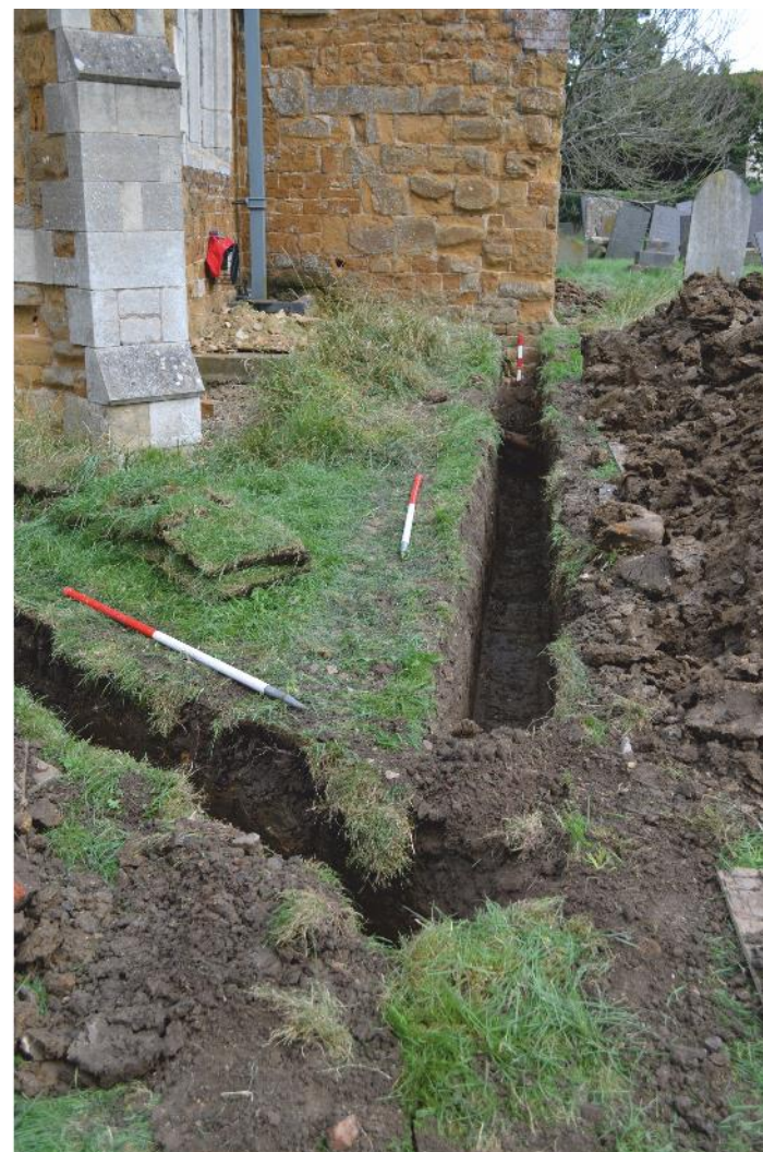
Pl. 26 Junction of pipe trenches from the south aisle and south porch, looking west. Scales 1m.
