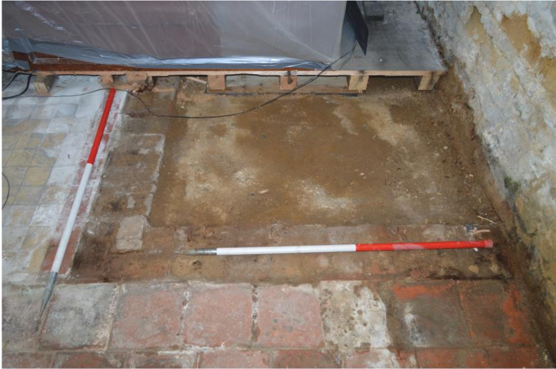
Pl. 21 North aisle floor area east of the organ after removal of old pew platform, looking west. Scales 1m
