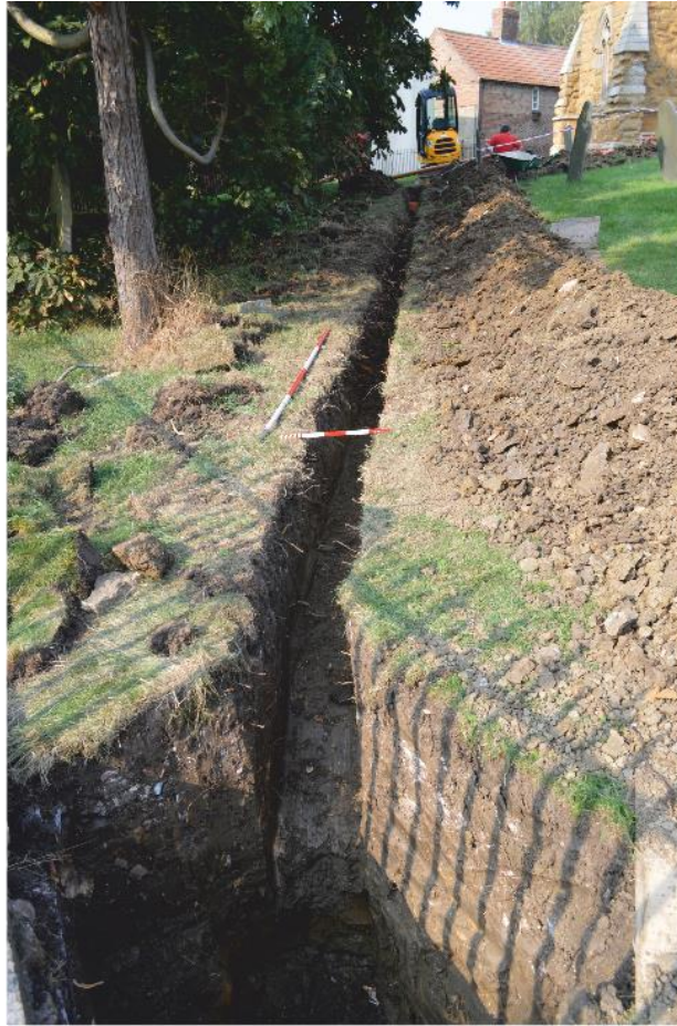
Pl. 29 View north-east along the pipe trench from the churchyard wall. Scales 1m
