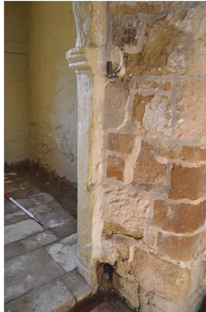
Pl. 6 South aisle door west jamb showing door pintle and pintle location at base, looking south
