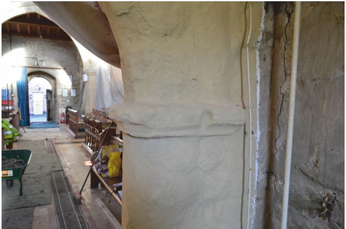
Pl 8 South door east impost, damaged.
