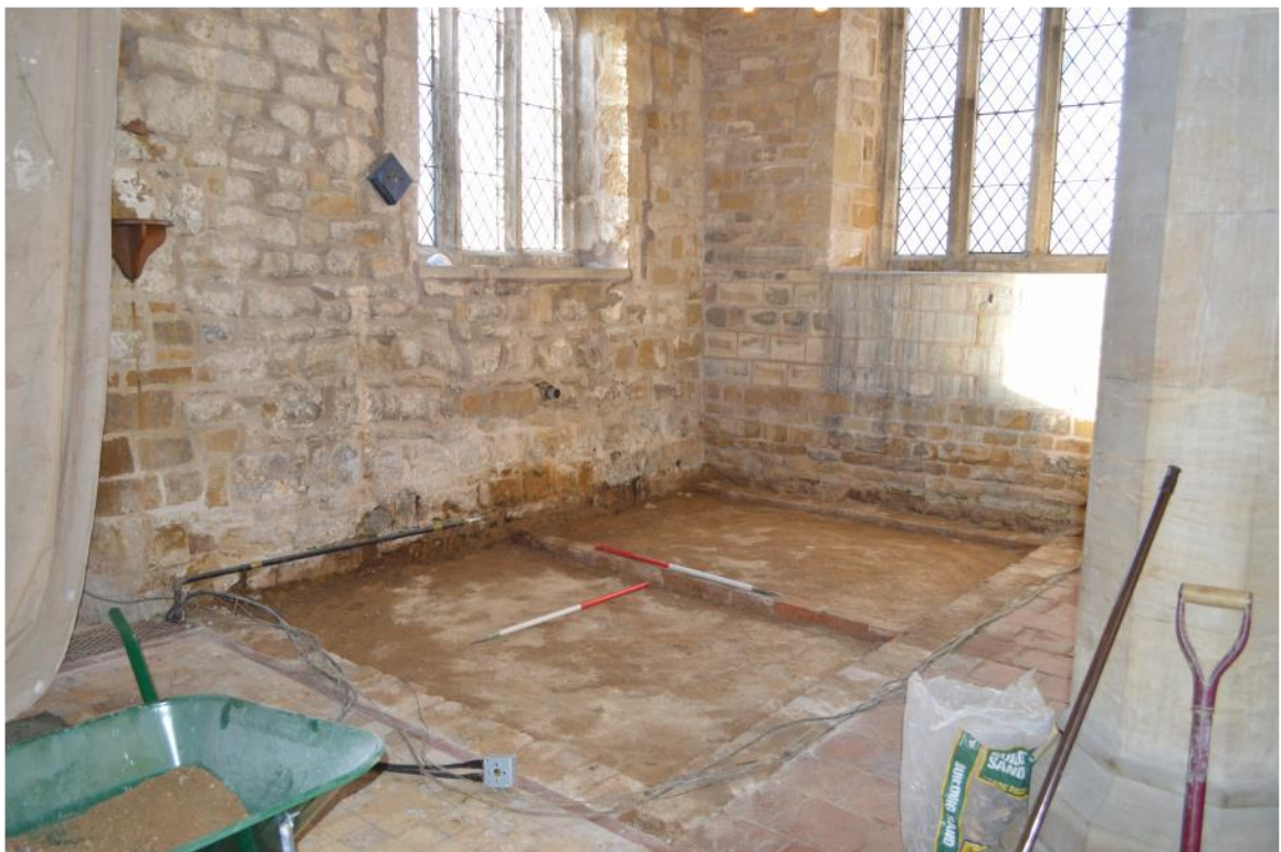
Pl. 4 South west corner of the south aisle after removal of the pew platform, showing brick sleeper walls. Scales 1m
