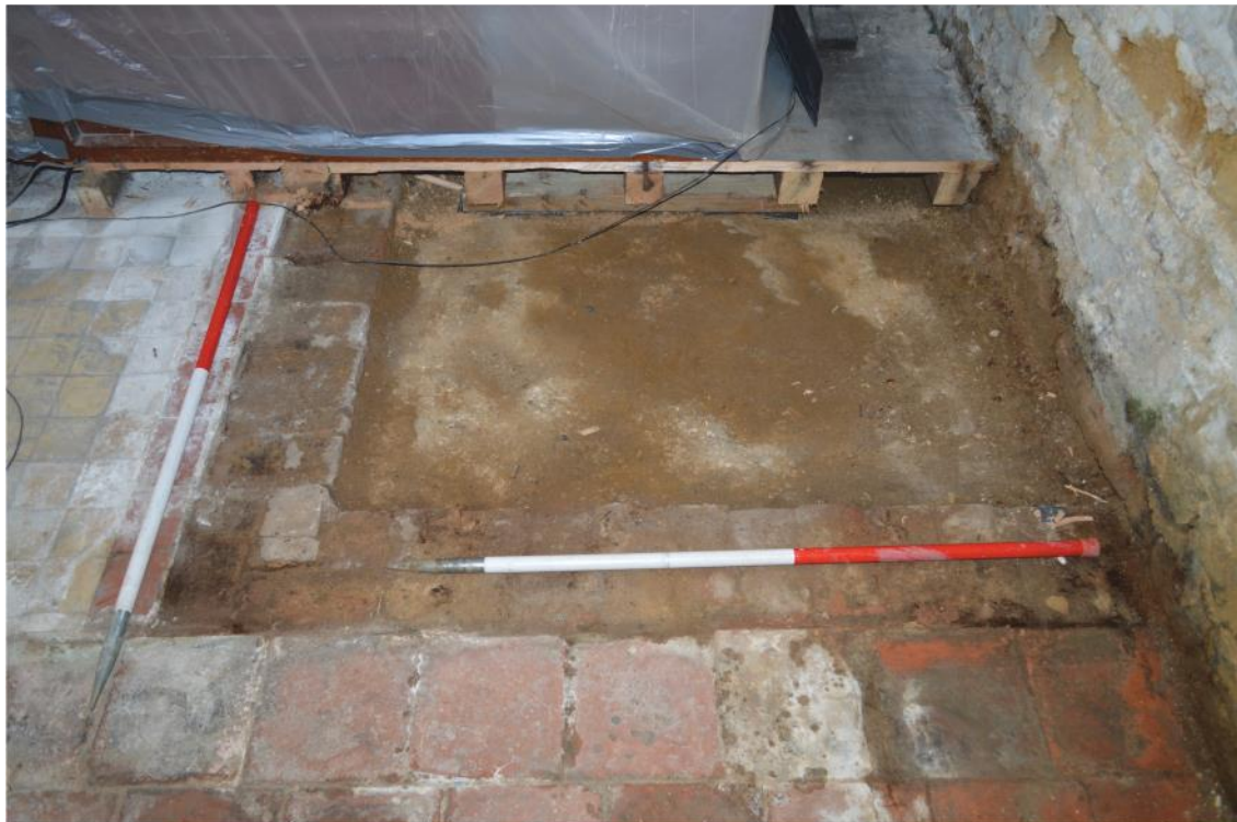
Pl. 16 North aisle floor area east of the organ after removal of old pew platform, looking west. Scales 1m
