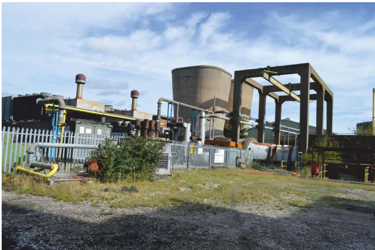
Pl. 17 Power plant with fan house and fan drift to rear, looking east
