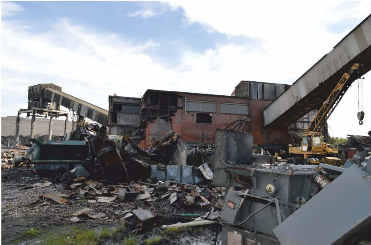
Pl. 19 ROM (run-of-mine) coal stock tower and gantry, showing demolition in progress, looking north-east
