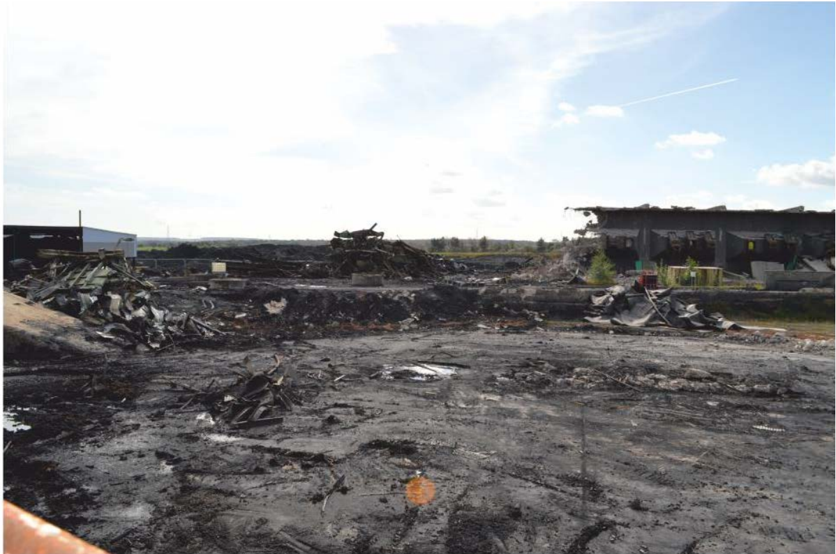
Pl. 21 Demolition in progress, looking east towards site of coal preparation plant at south-east corner of the colliery complex.
