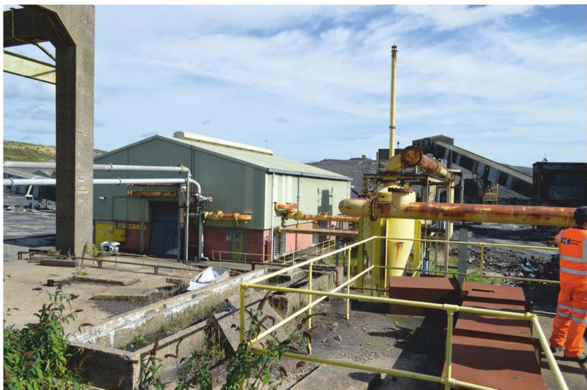
Pl. 18 Methane plant (to be retained)
