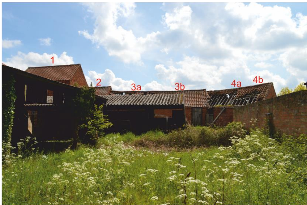
Pl. 6 General view of site looking south, from inside the crewyard showing buildings 1,2,3,4 behind modern open shed, with asbestos roof, not surveyed.
