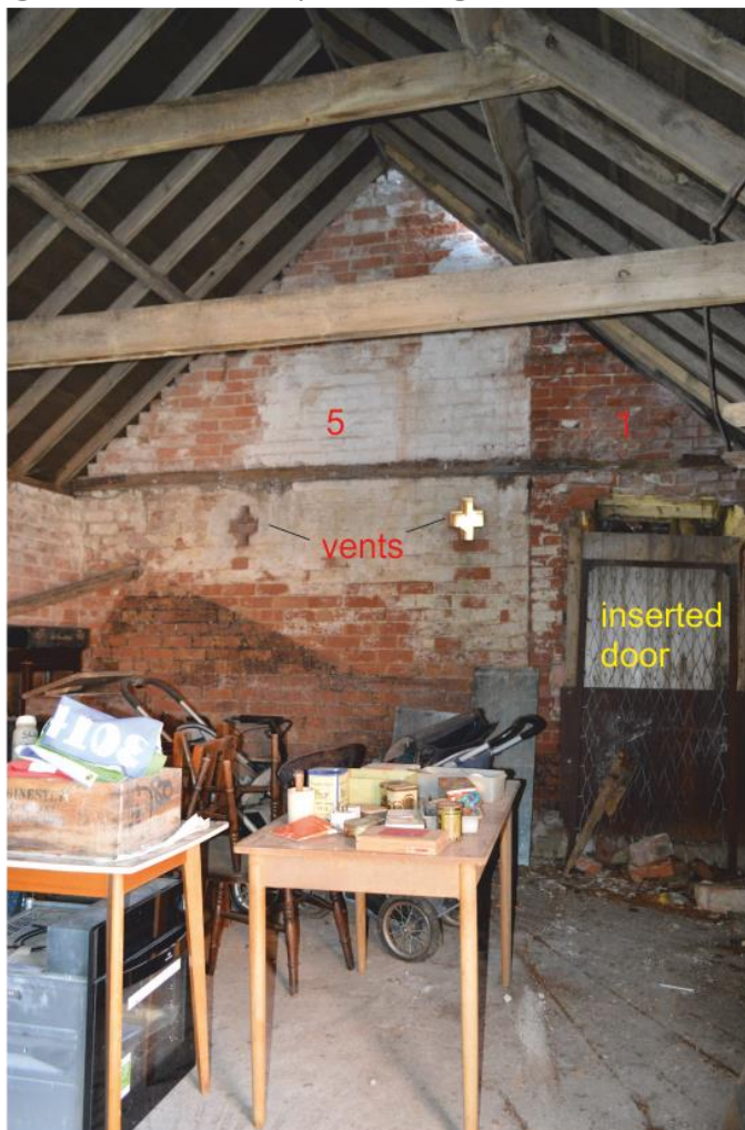
Pl. 40 Building 5 looking east. Inserted door to building 1 and machine sawn roof timbers
