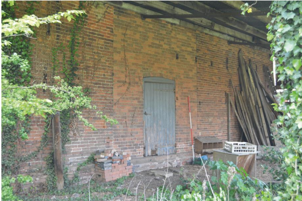
Pl. 47 Building 7, threshing barn, blocked door with inserted entrance on south-west elevation facing the crewyard
