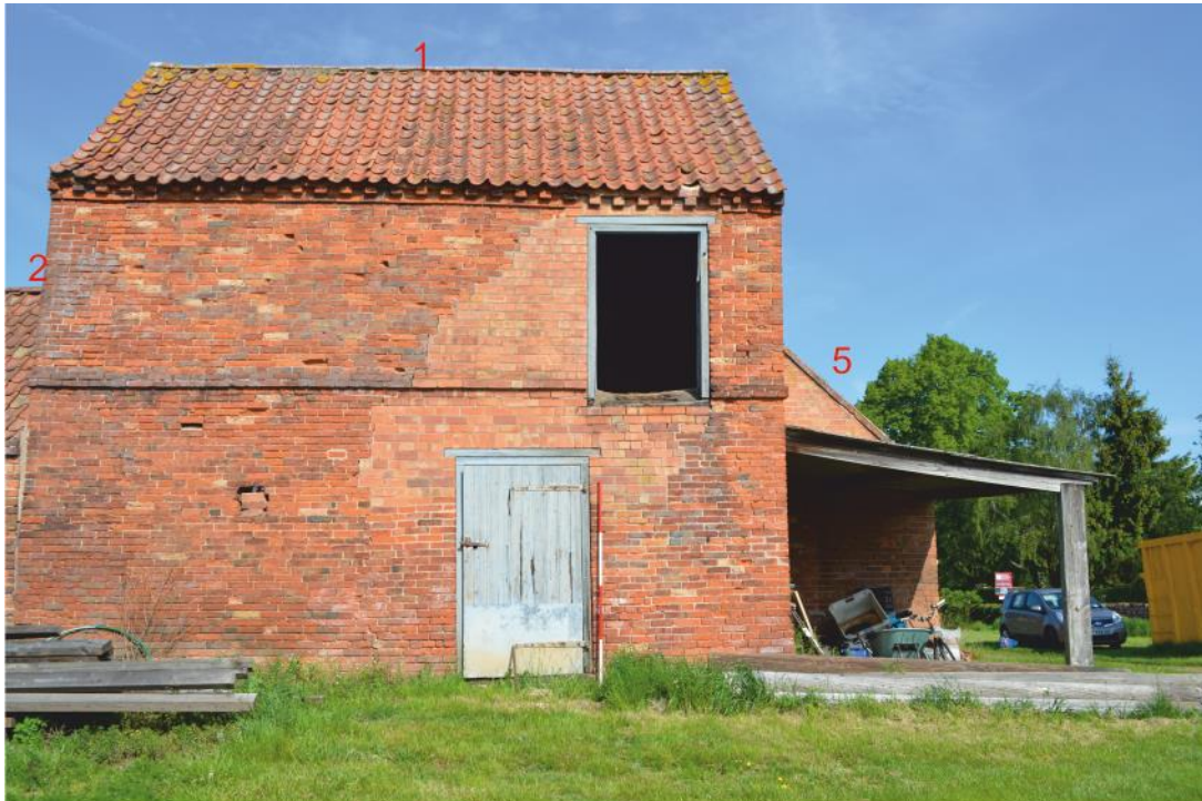
Pl. 11 Building 1, east elevation showing taking in door and repaired wall and door into area 1a.
