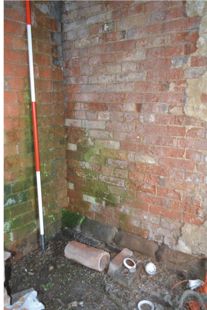
Pl. 42 Building 6 north wall (south wall of Building 5) built over stone chamfered plinth of Building 1
