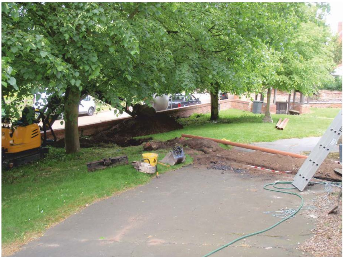
Pl. 8 General view of the service trench crossing the churchyard to the septic tank at the boundary wall of the churchyard, looking north-west.
