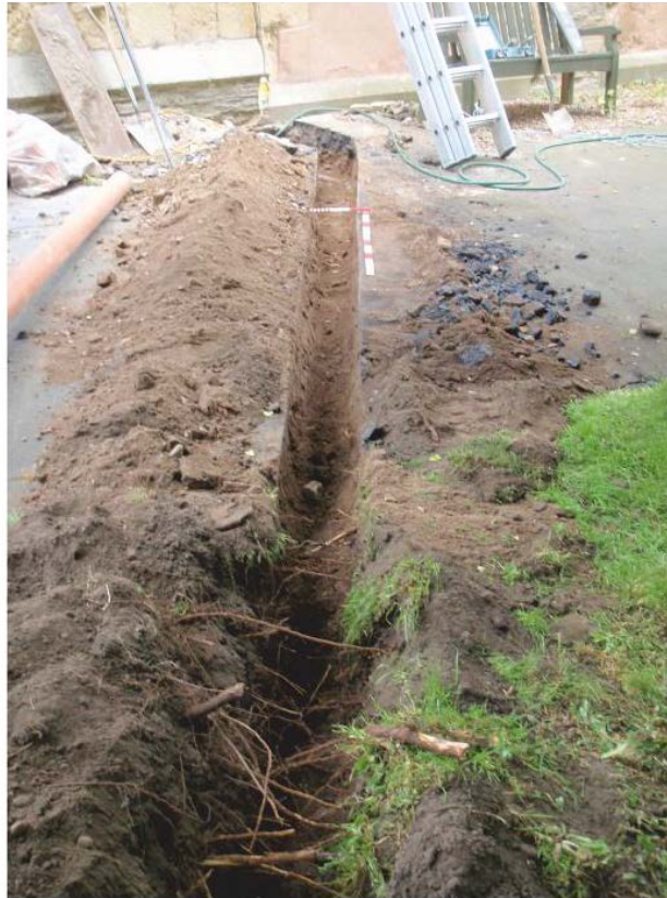
Pl. 7. Service trench running from the vestry to the septic tank, looking south-east.
