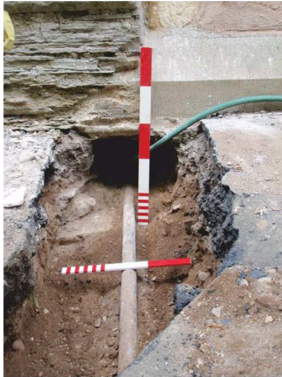
Pl. 5 The service trench at its exit from the vestry showing the vestry foundations and the pre-existing water and gas pipes, looking east. Scales 0.50m and 0.30m
