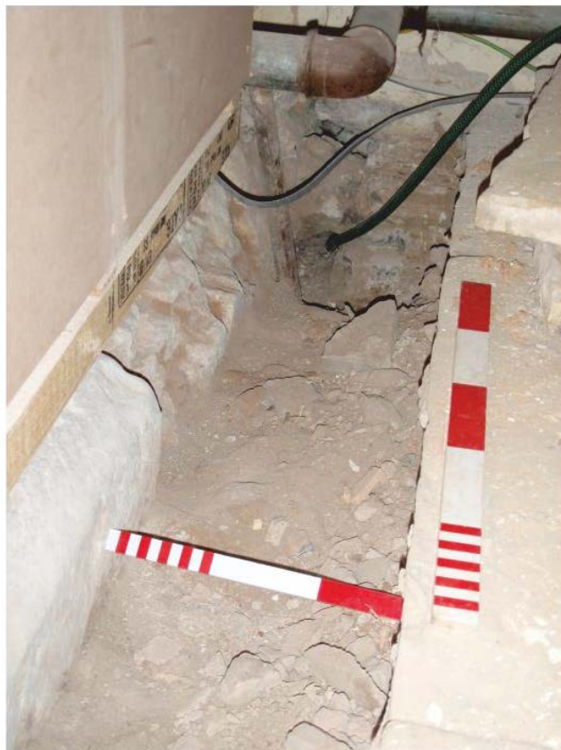
Pl. 4 The service trench at junction with west wall of vestry, looking west. Scales 0.50m and 0.30m.
