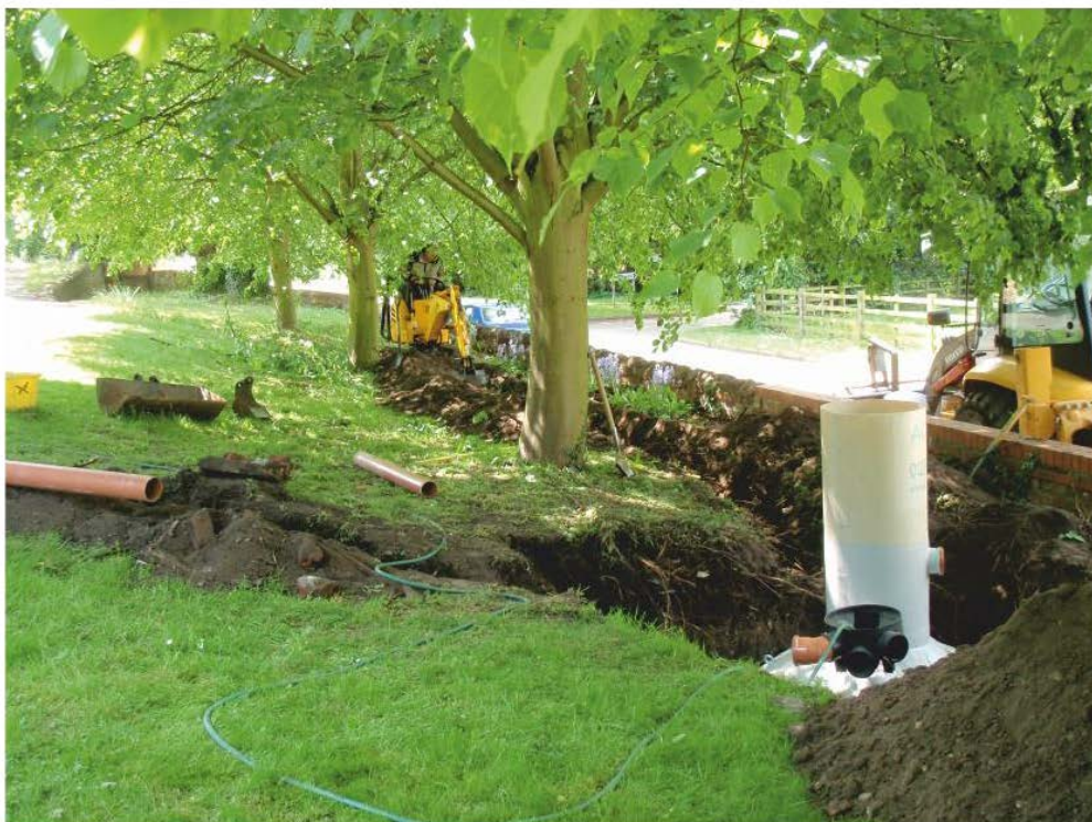
Pl. 10 General view showing excavation of the service trench south from the septic tank, along the churchyard boundary.
