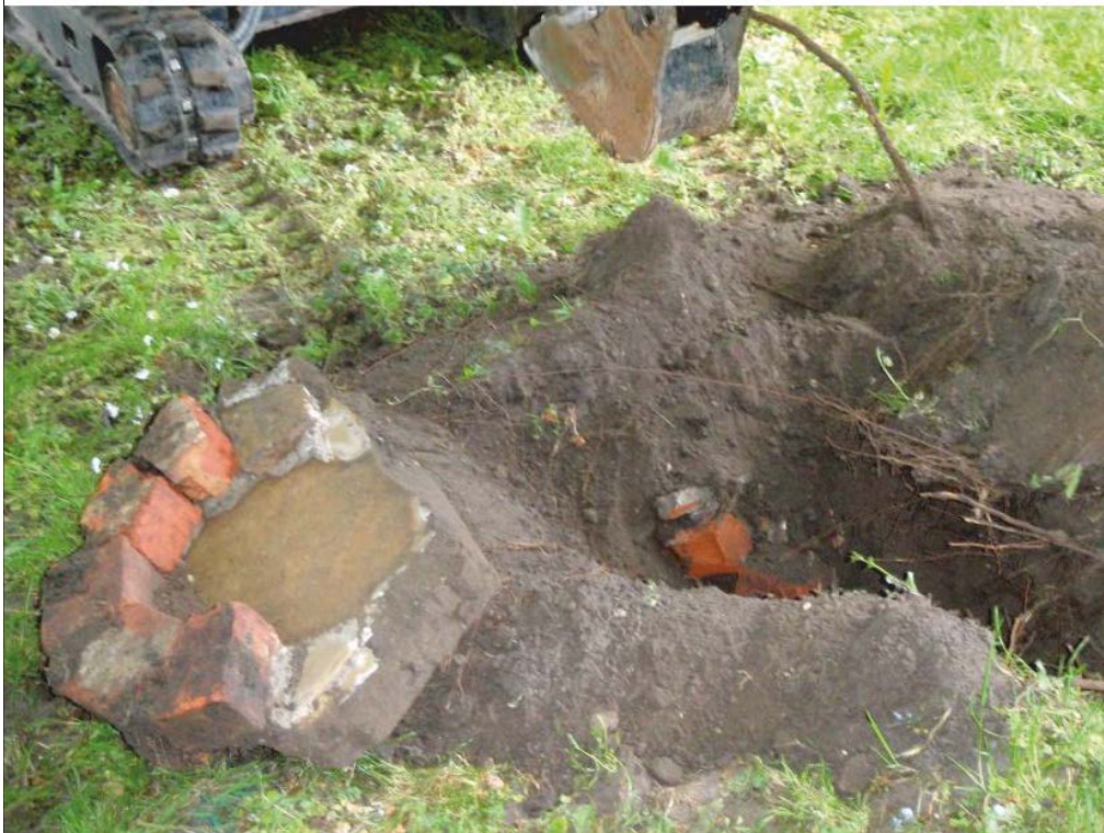
Pl. 6 Stone capping of old soakaway found in service trench west of the vestry.
