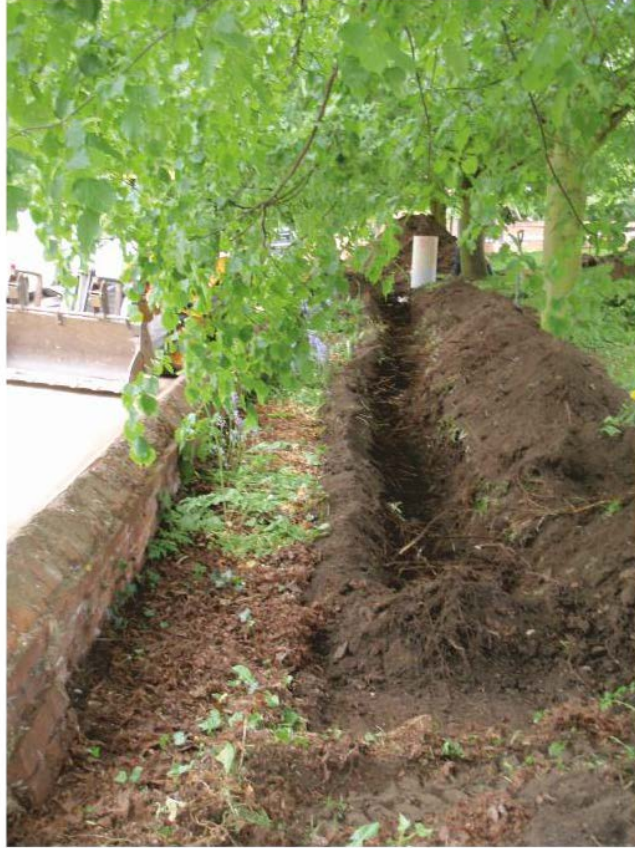
Pl. 11 Service trench along the churchyard boundary looking north towards the septic tank
