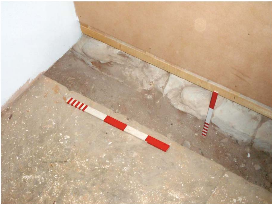
Pl. 2 Original plinth at the base of the tower north wall, revealed in the service trench in the vestry. Scales 0.50m and 0.30m
