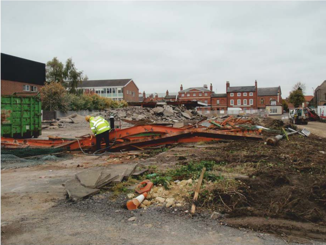
Pl. 1 General view of the bus station during demolition and clearance of the site, looking north
