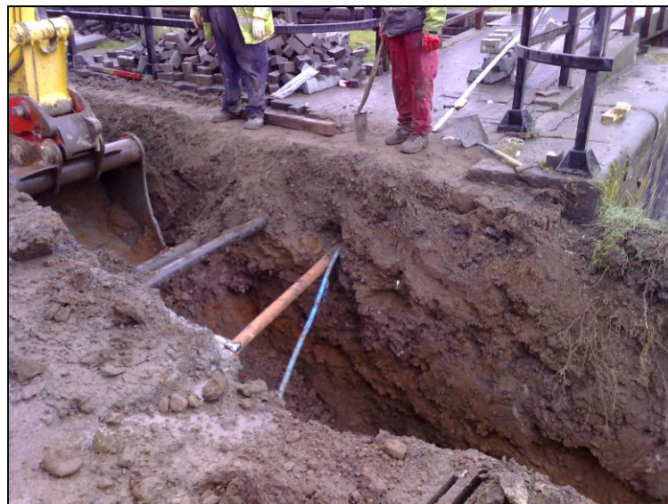
Figure 23: Location of services at the foot bridge looking NNW
