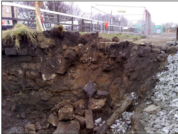
Figure 17: The revetment wall after it collapsed
