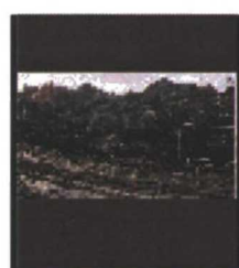
PID: 11869 (1057-50 - print 2004-62-18) Stone blocks excavated during pile driving, dock site, east of Shipyard Road. (54265 bytes)
