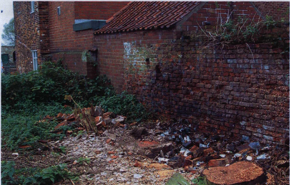
Plate 4 - Brickwork and associated floor surface along eastern perimeter, with dump of nineteenth-century ceramic and glass, at site of structure shown on 1893 OS map.
