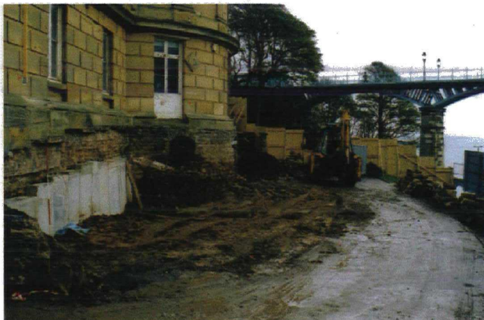
Photograph 7 – following complete excavation showing natural Clay level with footpath and cellar floor. Scale 2 metre
