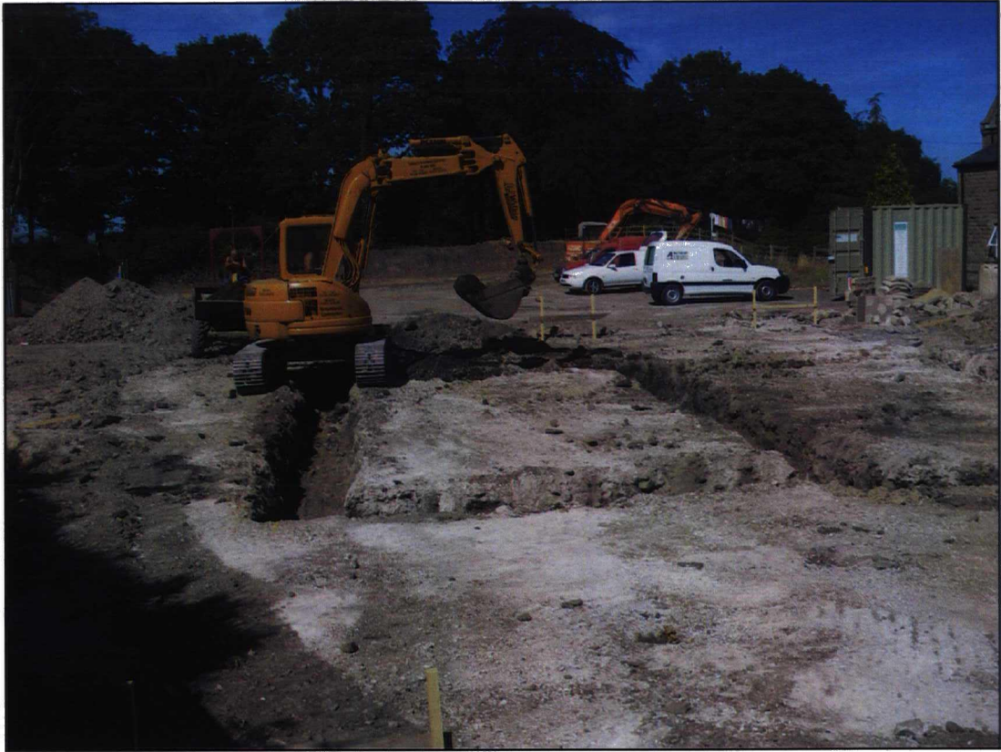
Plate 1: Plot 4 during excavation looking north-east, once tarmac and hardcore layers had been removed.
