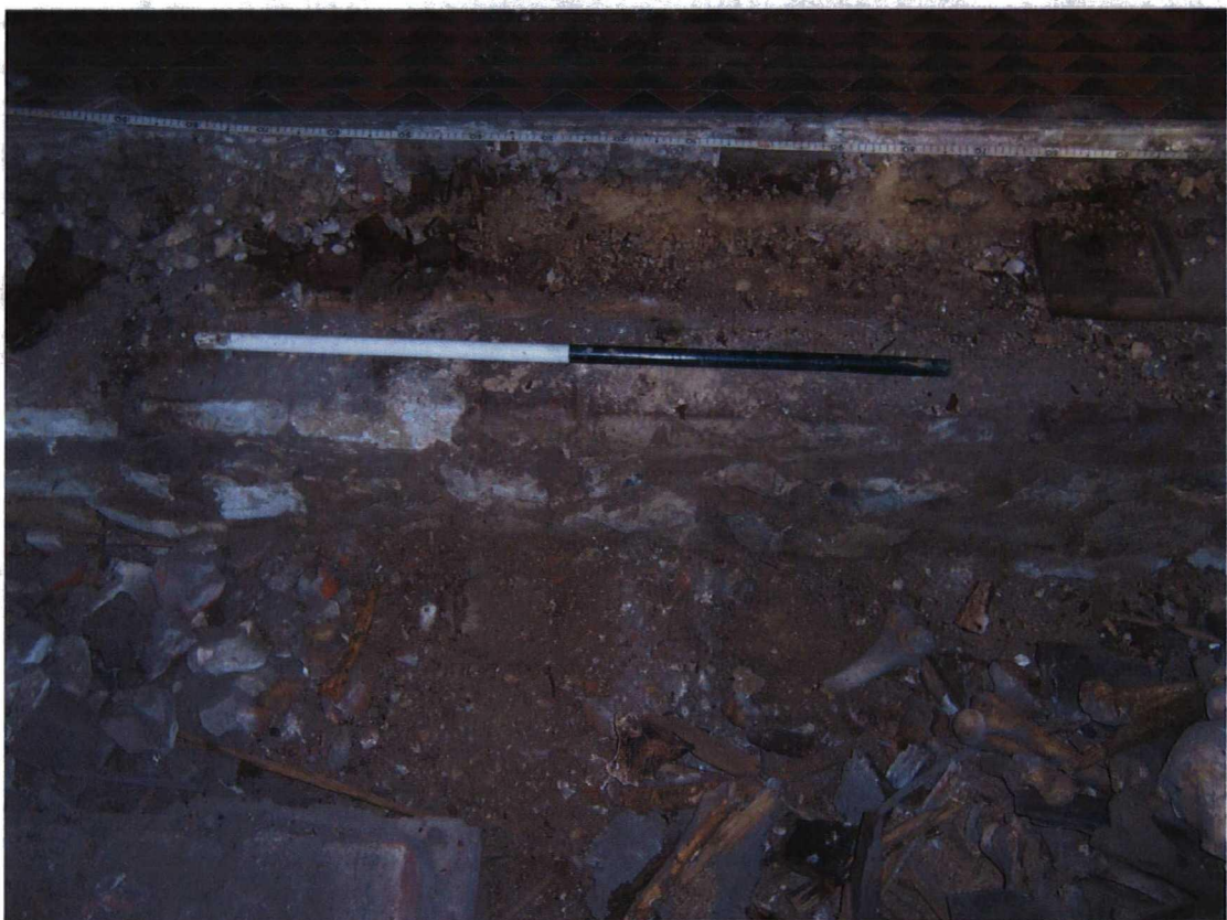
Plate 10 Northern limestone foundations (2005), with later brick repairs (2004), underlying the nave flooring (2001) within the southern pews. Viewed from the south.
