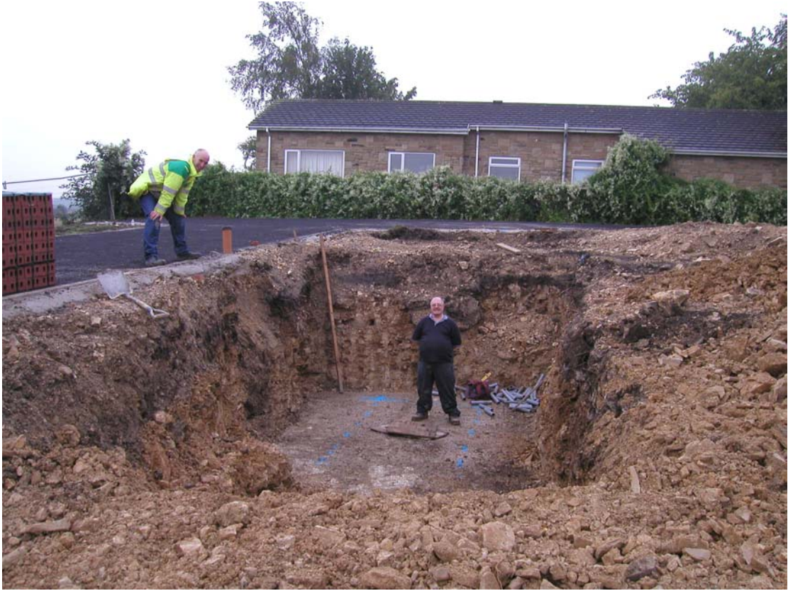
Plate 7 The large soakaway
