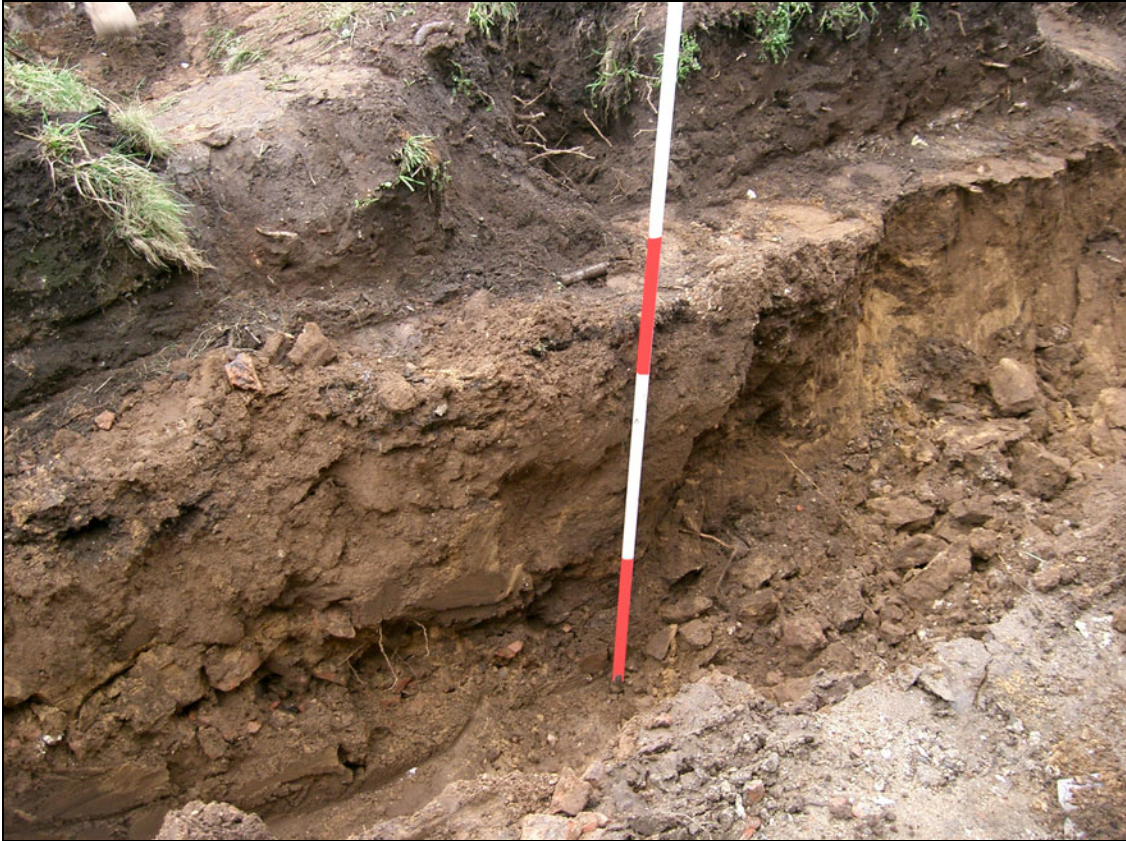
Figure 4 Pit number two immediately after collapse (note bricks in base of footing)
