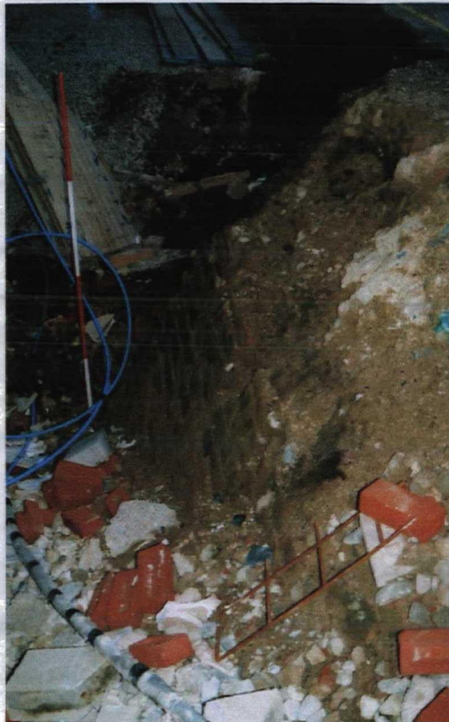
Figure 2 Film 2 frame 28a Showing the top of the wall in relation to the building Scale 2 metres in 500mm divisions
