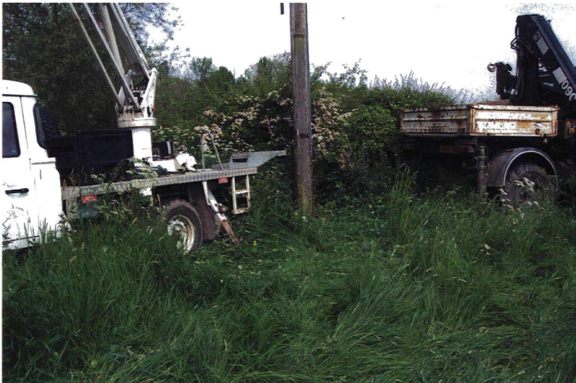
Plate 2. View of Pole 1, Prior to the Cutting of the Pole. Facing North
