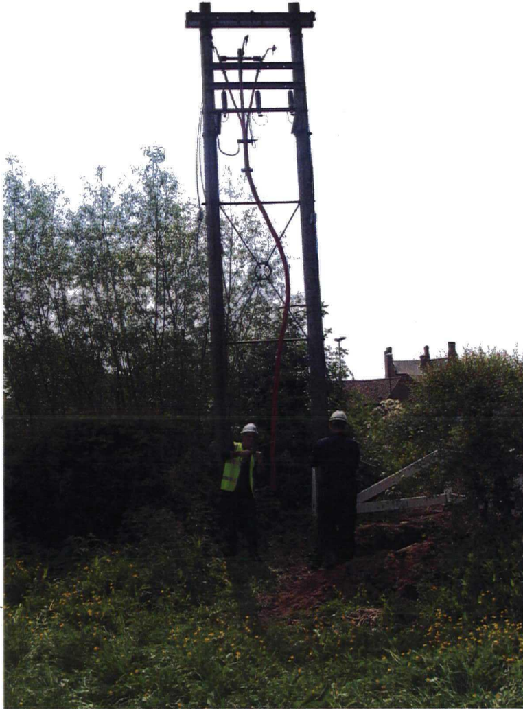
Plate 5. Poles 2 & 3. Facing South West
