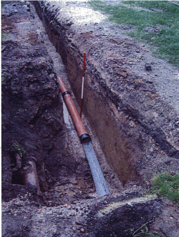
Plate 3. Overall View of Services. Facing North East
