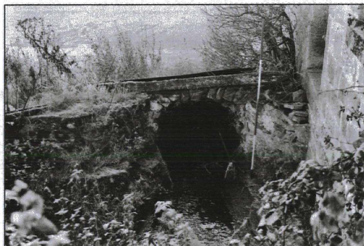
Plate 6 (143: 1/19) exterior, north elevation: view of the spillway at the foot of the phase 4 and 5 corn mill
