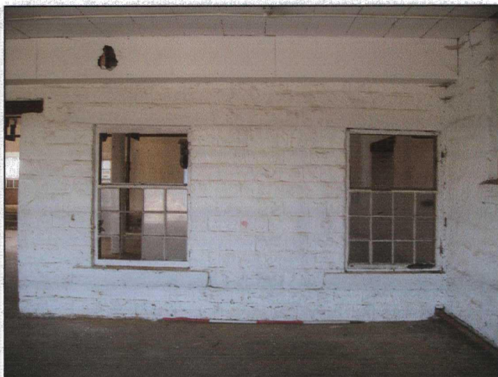
Plate 65 (20: 2/20) Room 1/7: view of the type 3 windows in the phase 1 'exterior' elevation = south wall, from the north
