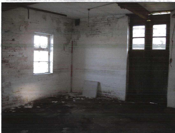
Plate 73 (78: 4/27) Room 2/2: general view of the additional loading door in the east wall, from the south-west
