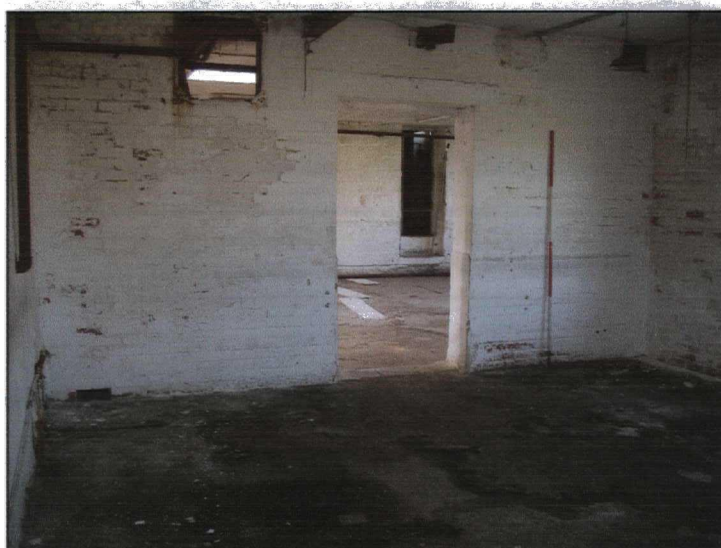
Plate 74 (77: 4/28) Room 2/2: general view with bearing box to the upper wall in the top of the wall that predates the sprinkler system, from the south-east
