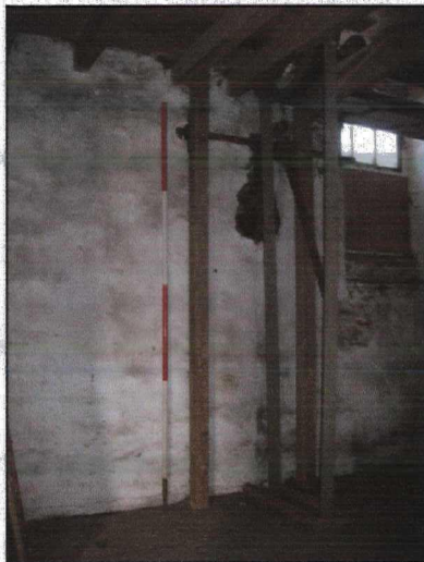
Plate 76 (90: 4/14) Room 2/3: view of the pulley with in situ belts, from the south-west
