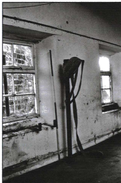
Plate 71 (101: 4/3) Room 2/1: view of the in situ sprinkler system with attached hose, from the north-east
