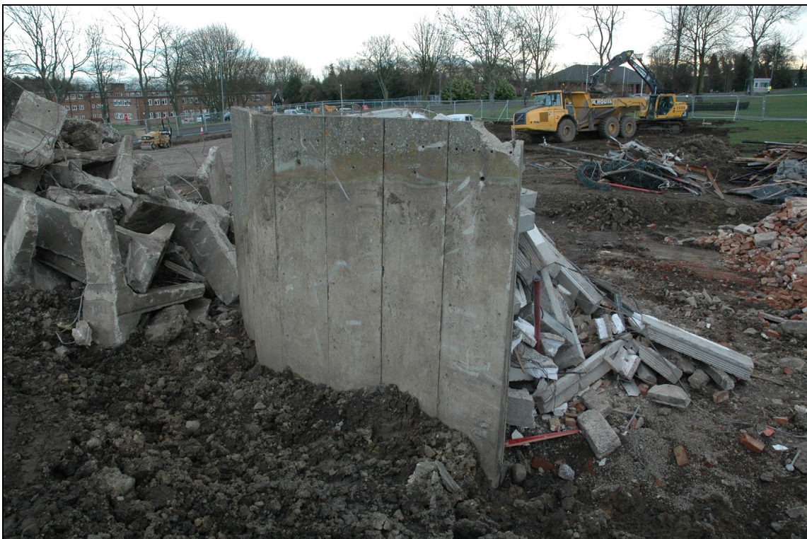
Figure 52 Bunker, 50; the turf line can still be seen on the outer face of the section of blast wall
