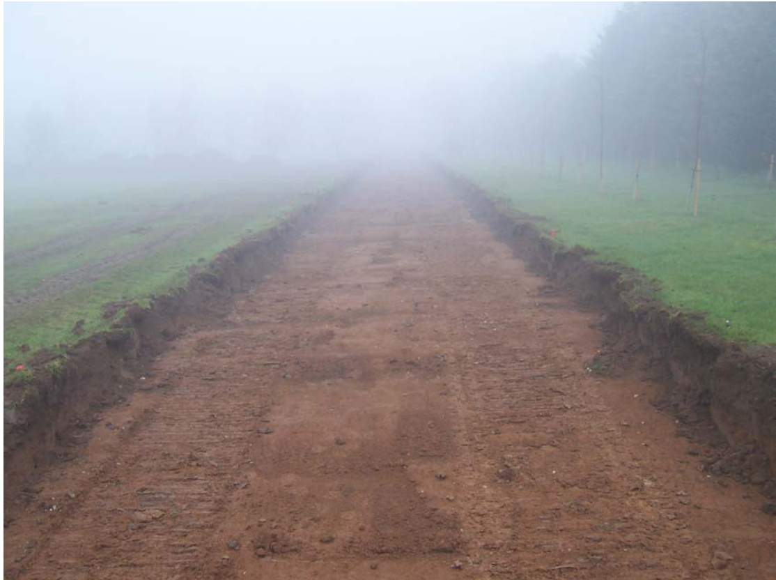
Plate 5 The road strip along the north-south longitudinal section, showing deposit (105) underlying deposit (101), looking north.
