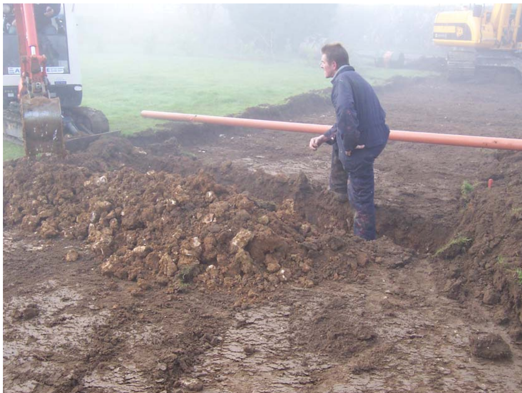
Plate 10 Showing the excavation of a cable trench across the southern section of the road. Deposits (102) underlying (105) were noted in this section of the works. Viewed from the northeast.
