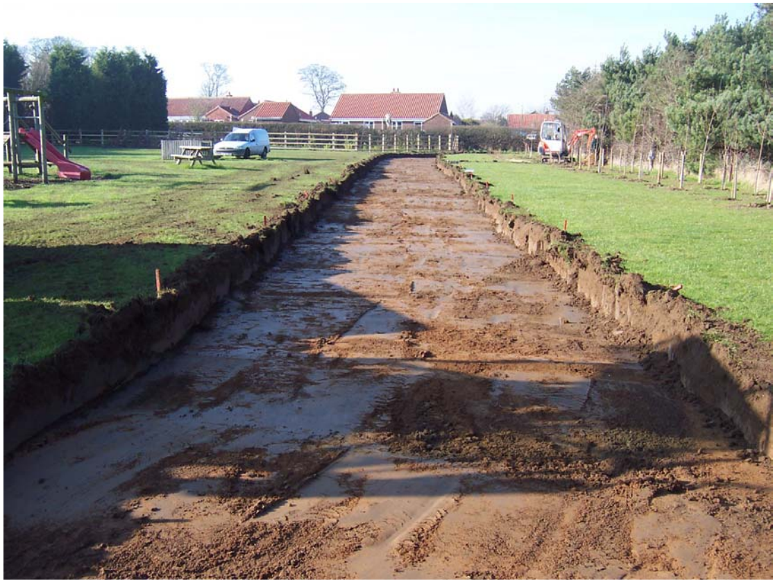
Plate 4 The road strip underway at the north end of the site, showing hillwash/subsoil (105) underlying topsoil (101), looking west.
