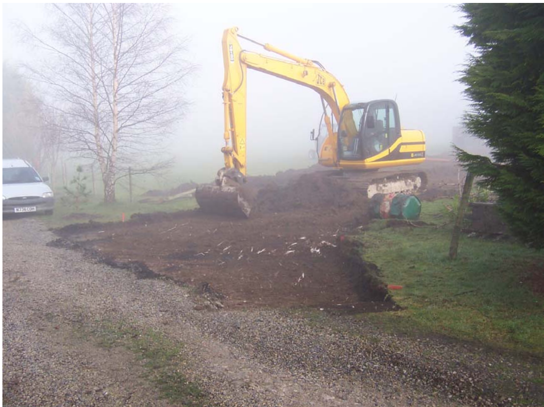
Plate 6 The road strip at the southwestern corner of the site, showing topsoil (101) overlying (105), looking northeast.
