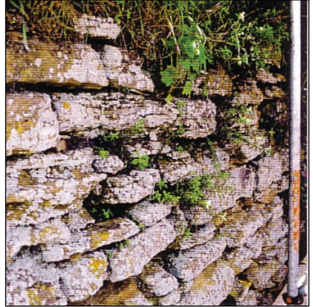
Plate 39: Lichen Diploicia canescens on the lower level of the east external elevation.
