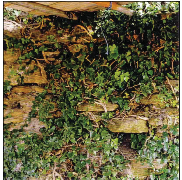
Plate 43: Ivy stems and loose masonry 7.5m above ground level.
