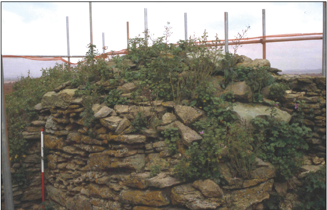
Plate 37: Vegetation at the top of the north-east tower, prior to consolidation.
