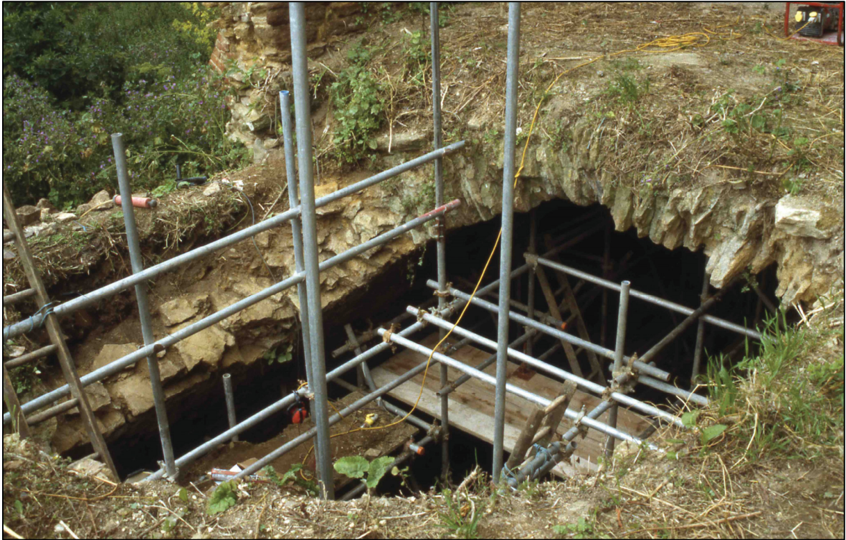
Plate 17: Hole in basement vault, prior to consolidation, looking north-west.
