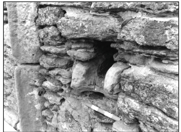
Plate 27: External spout from sink in north wall of uppermost room, adjacent to vertical string course, looking E.
