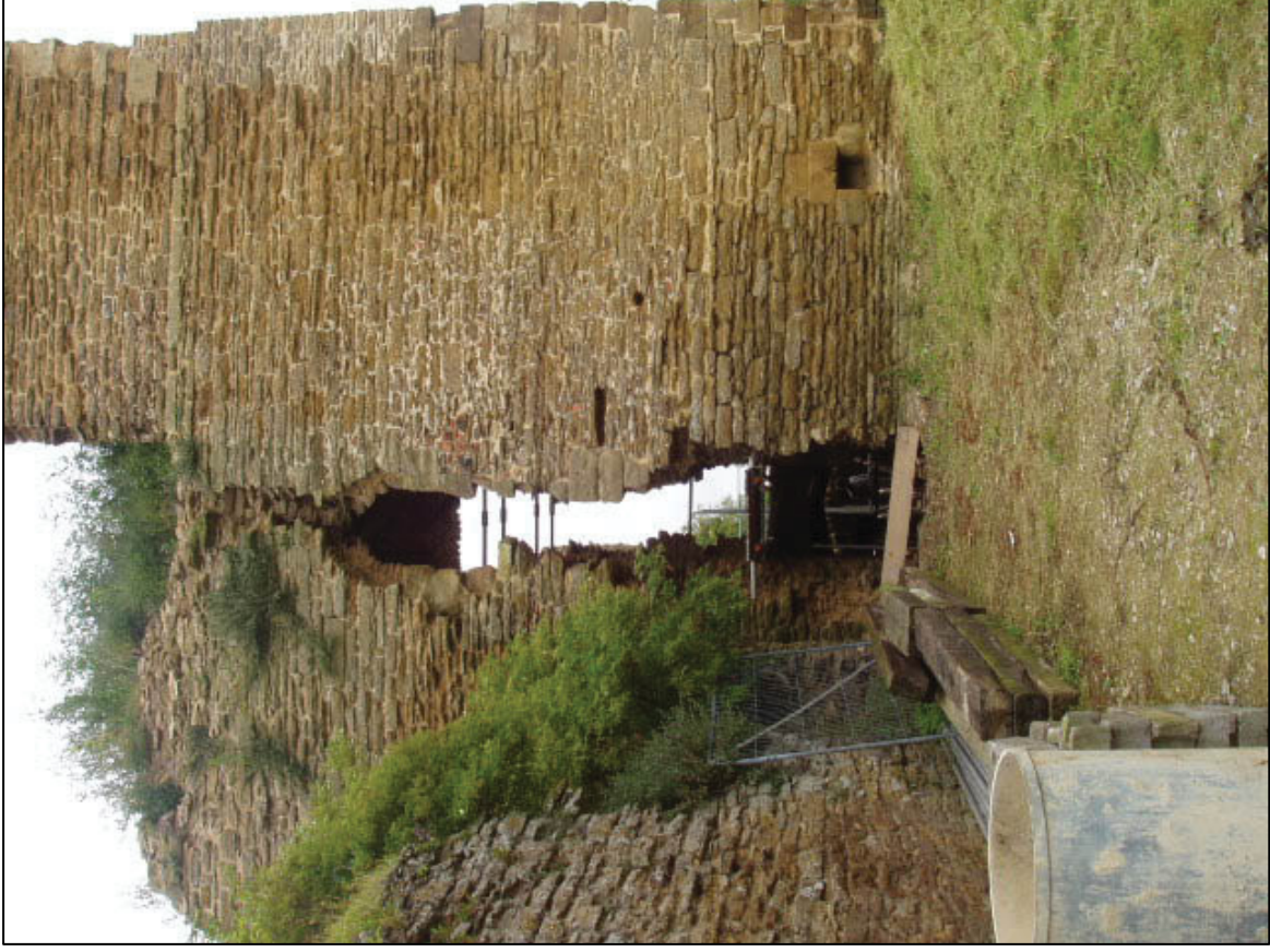
Plate 16: Lower part of north external elevation, showing crack over window W2/3, prior to consolidation, looking S (May 2002).
