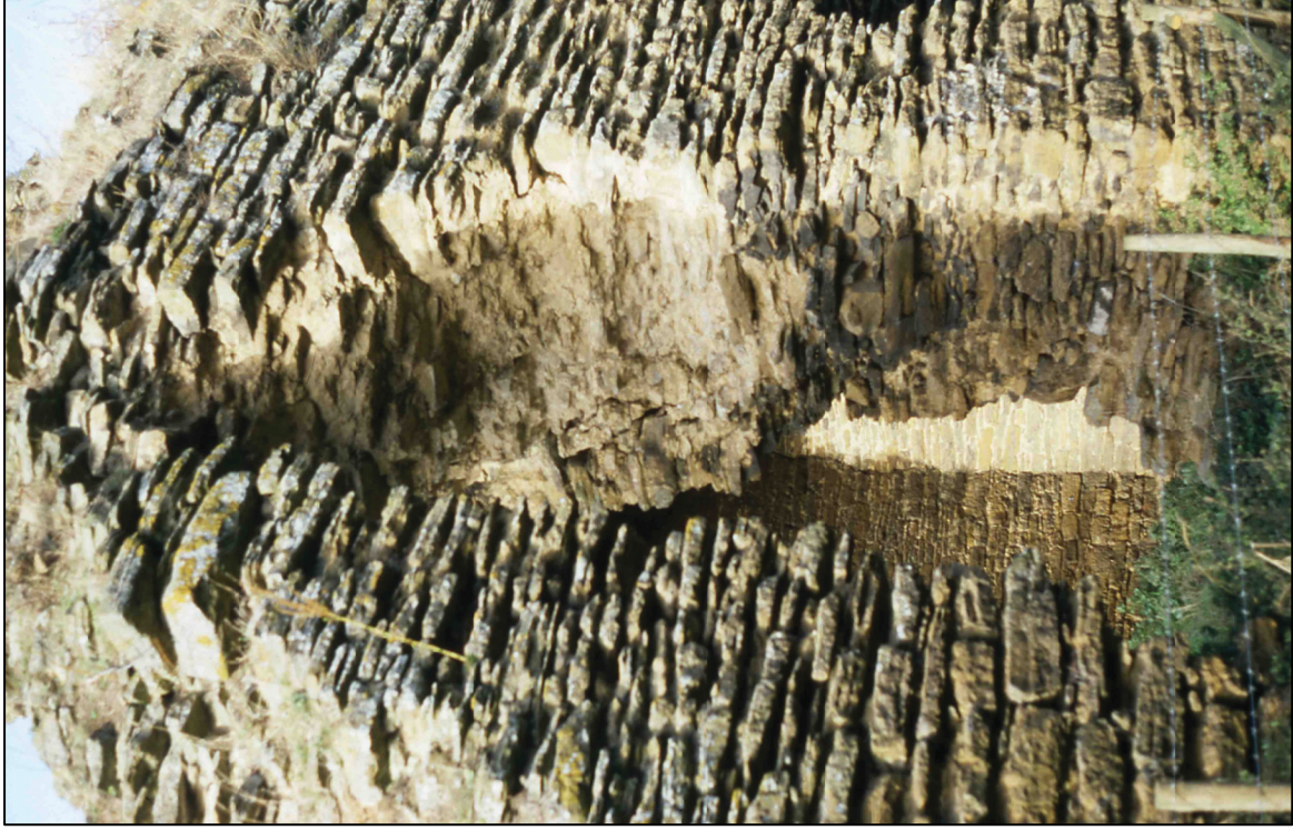
Plate 15: Area of collapse, east external elevation, prior to consolidation (September 1996).
