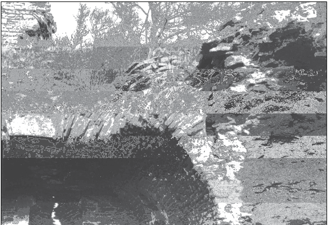
Plate 14: South edge of ground floor vault, showing fracture, looking NE (September 1997).
