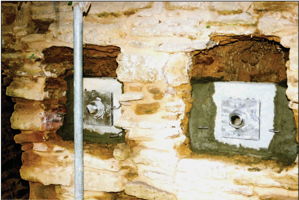
Plate 48: Inserted anchors to support structural ties running across the ground floor space.
