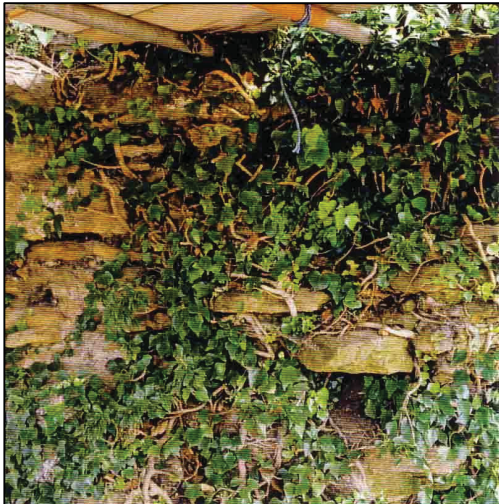
Figure 4 Sheriff Hutton Castle: ivy stems and loose masonry 7.5m above ground
