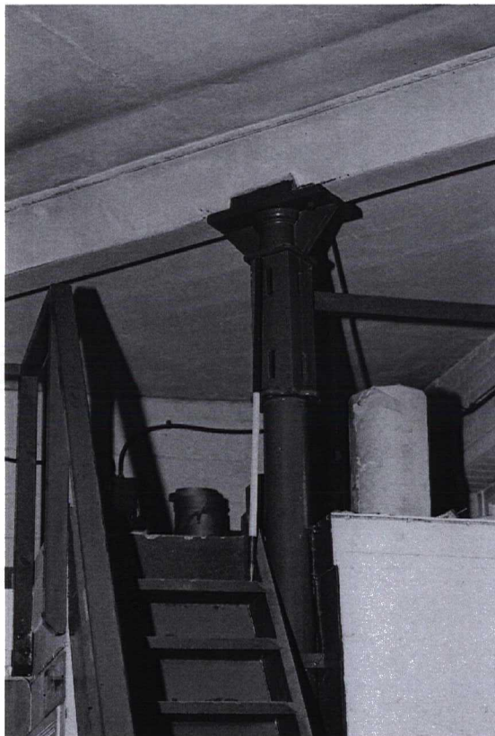
Photograph 34 9985/26 SE The top of a cast-iron column where it is bolted to the beam. Note the single bolting face for a drive shaft hanger
