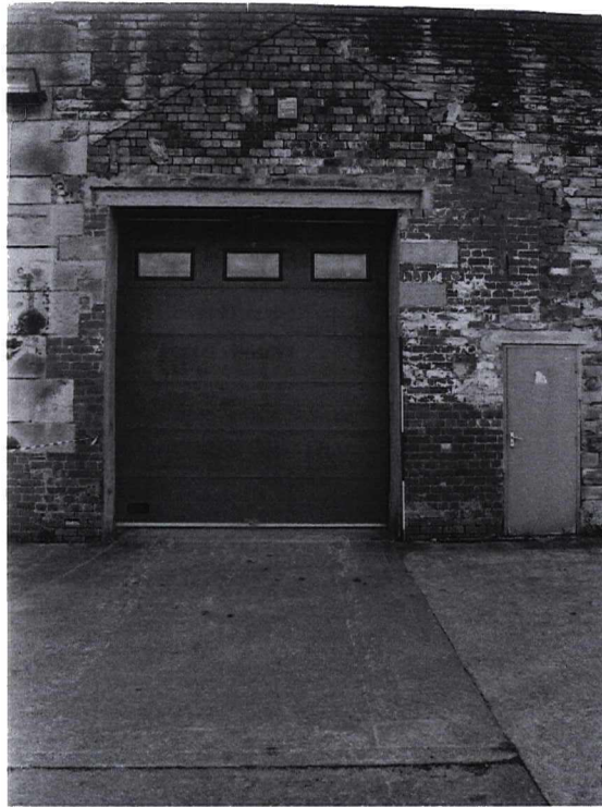
Photograph 23 9984/2 N Modern roller-shutter door. Note the encased gable wall and brick infilling
