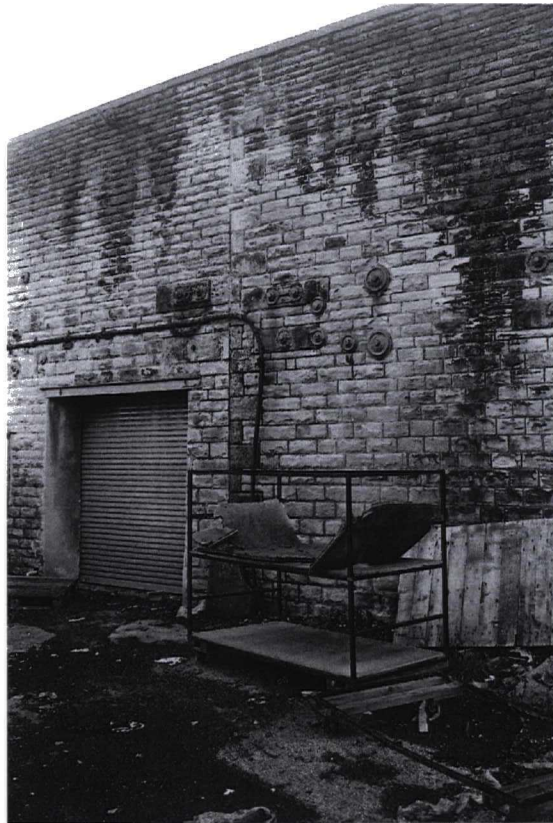
Photograph 19 9984/6 NW Wide roller-shutter door with straight joint to the side
