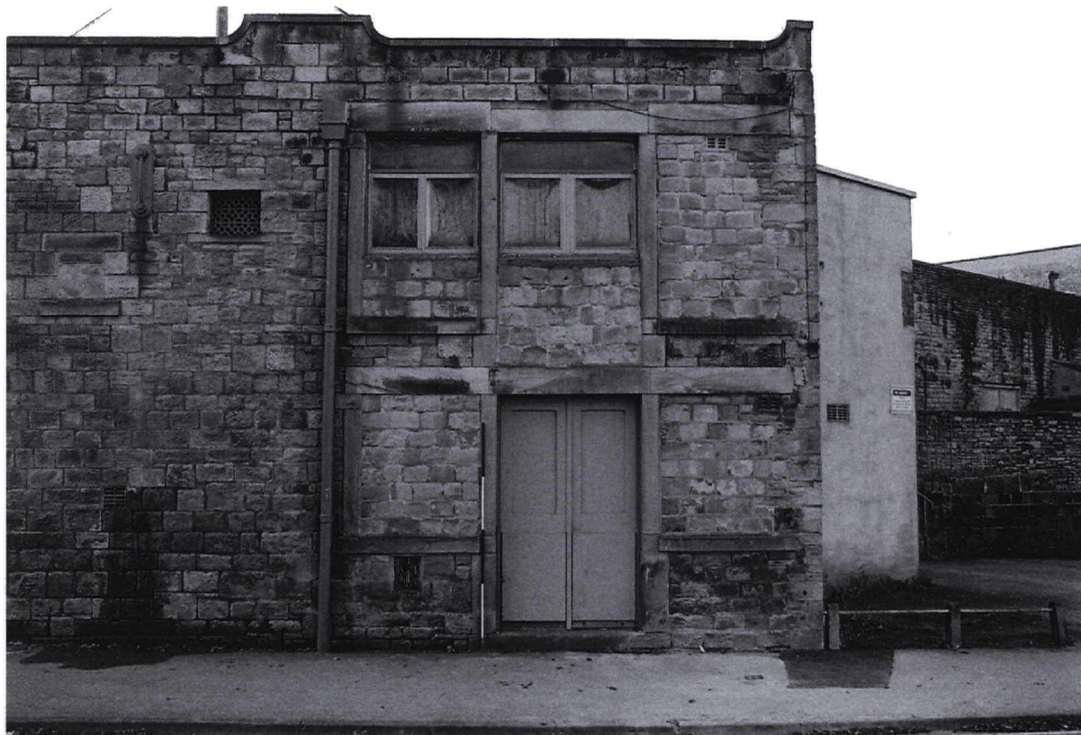
Photograph 1 9984/19 NE Ground-floor double door and first-floor double windows. Note the early blocked opening to the side of the doors
