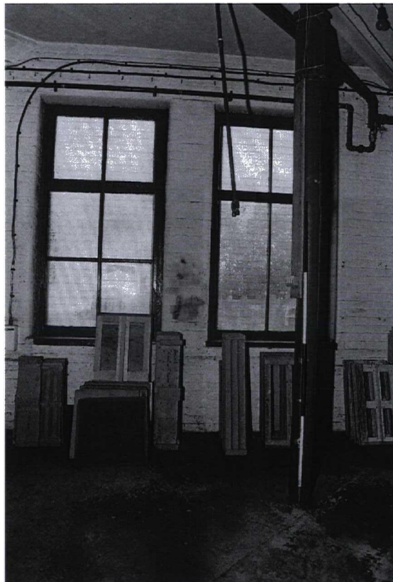
Photograph 38 9985/27 SW A cast-iron column in the foreground and a pair of two-over-four, top-opening, case- ment windows beyond
