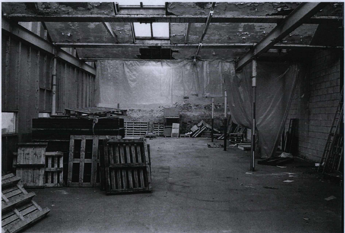
Photograph 62 9984/36 N View showing cast-iron columns and roof-lights. Note the internal partition on the left
