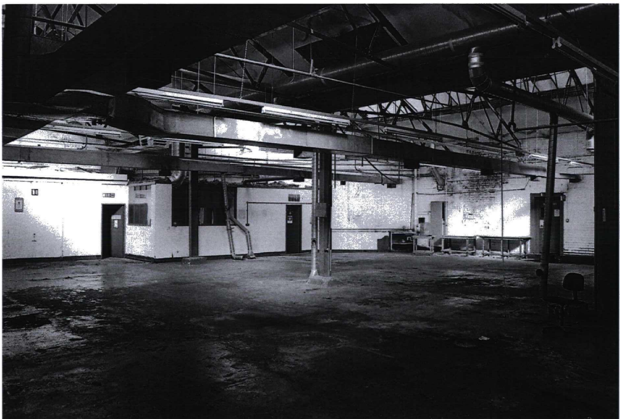
Photograph 46 9983/23 SW General internal view showing steel, 'T' section stanchions and the ventilation system
