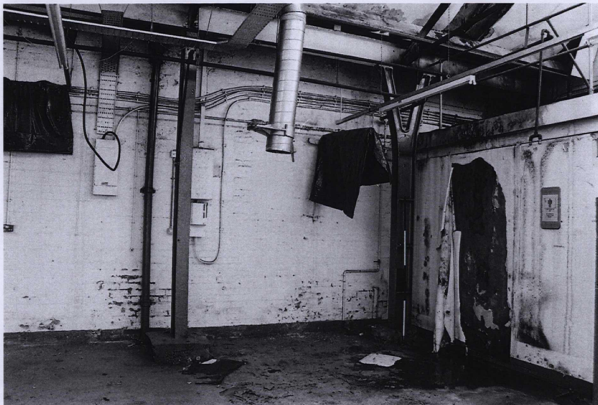
Photograph 77 9983/26 E Cast stanchion with 'Y' shaped head
