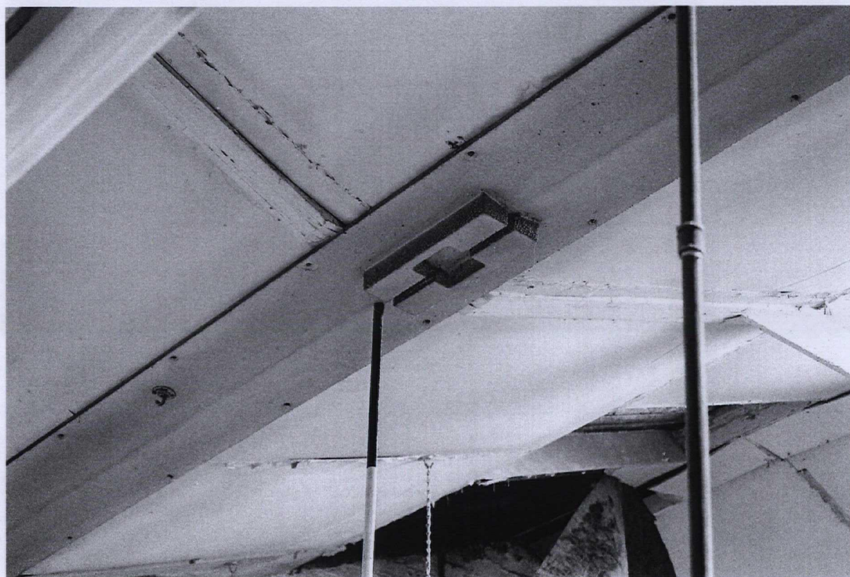
Photograph 78 9983/19 N Former position of a drive shaft hanger
