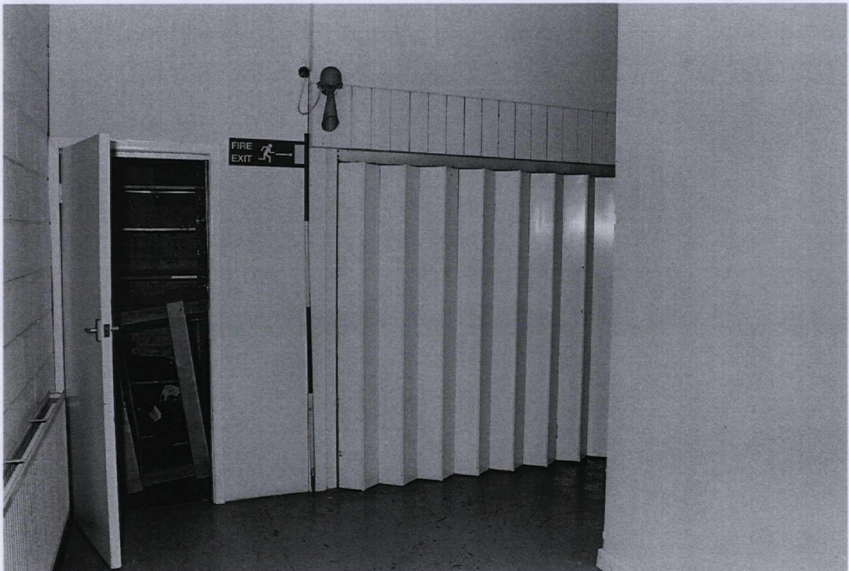
Photograph 94 9985/15 SW Lift doors
