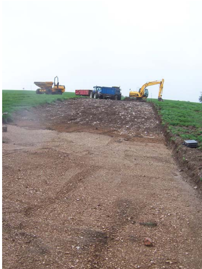
Plate 2 Initial topsoil stripping at the site showing underlying natural deposits (in order from foreground) (102), (104) and (103). Note the varied topography, looking southwest. 1m scale.
