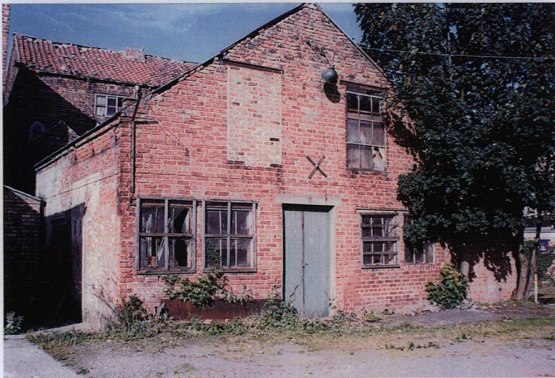
PLATE 2 REAR OF 2A-4 CASTLEGATE, SHOWING OUTBUILDINGS AND DECAY ON MAIN BUILDING
