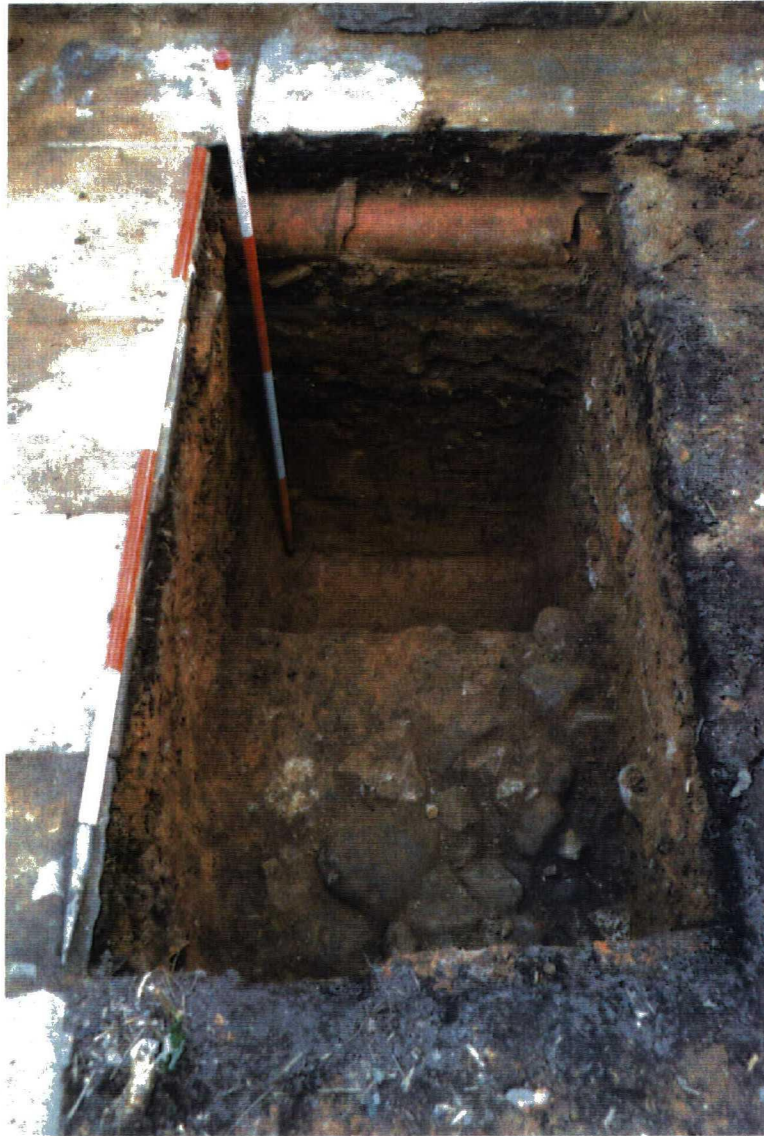
Trial Hole No.3, as excavated, revealing the depth of the natural sand deposits.
