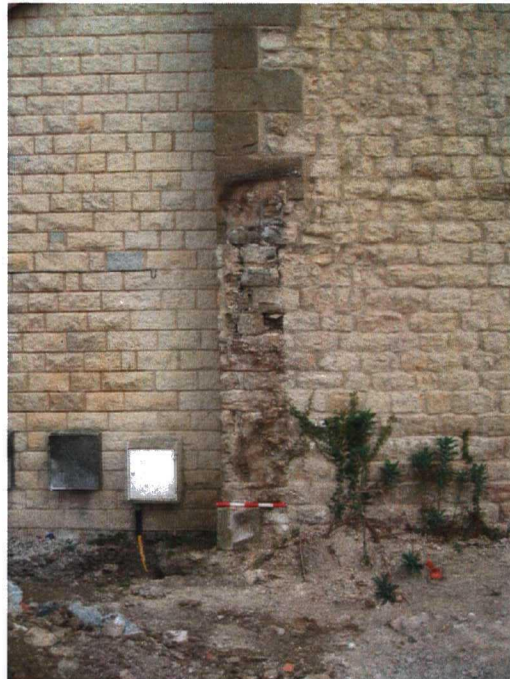
Plate 3 Wall scar on NW corner of former Meeting House, looking E (walling to left is 20 th century extension)
