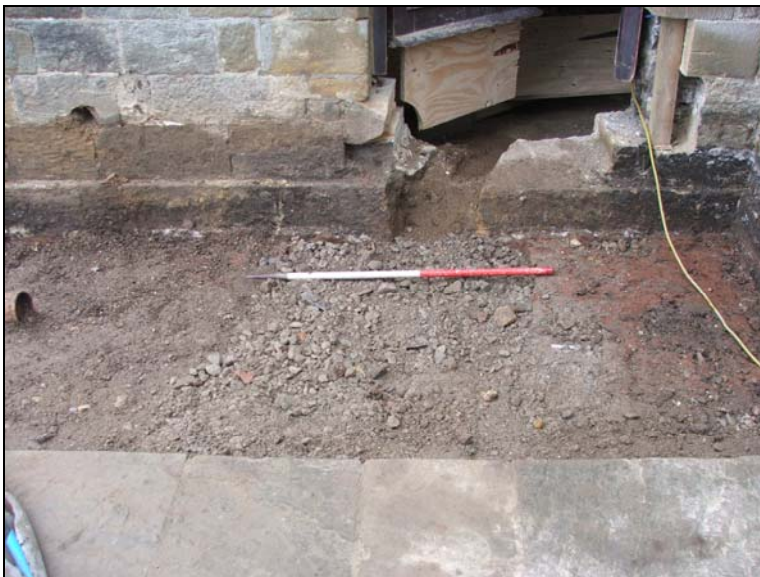
Figure 19: Lodge step area showing cut through Lodge wall of pipe. Looking east.
