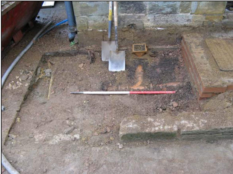
Figure 18: Lodge step under excavation showing modern drain and other service disturbance. Looking east.
