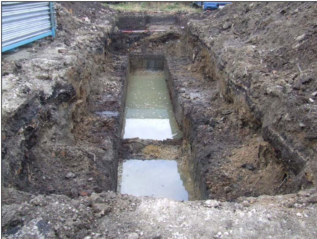
Figure 5 Trench 2, facing north. The very loose nature of the dump deposits is obvious
