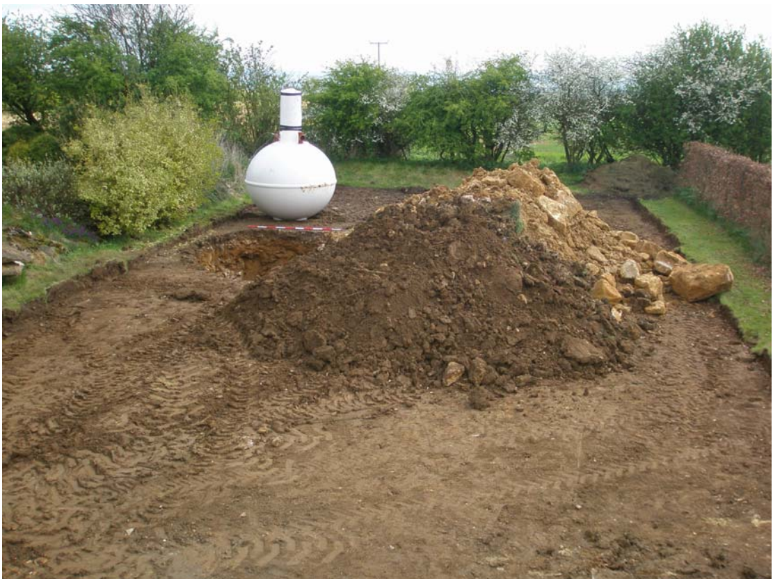
Plate 4 The topsoil stripped area and the first septic tank (klargestær) installation, viewed from the north
