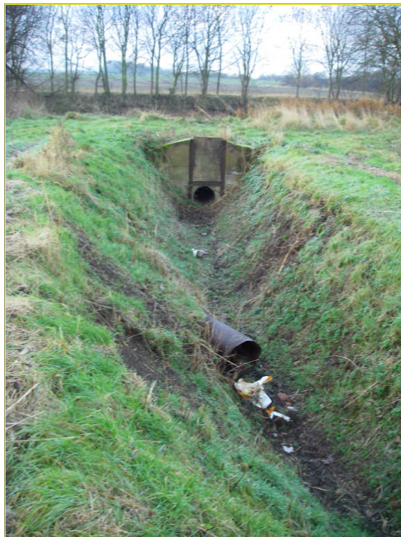
Photograph 4 – Northern drainage ditch showing sluice gate at western end, viewed facing southwest
