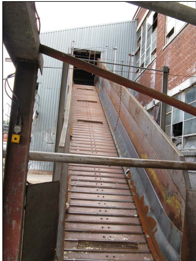
Figure 17 Western conveyor leading to underground tank
