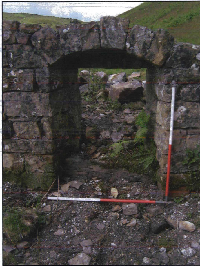
Plate 9. Opening at north end of western wall during works, looking west. Scales 1m.
