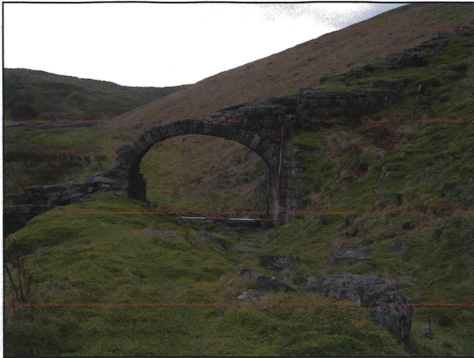
Plate 3. East side of arch over track-way before works, looking west, scale 2m.
